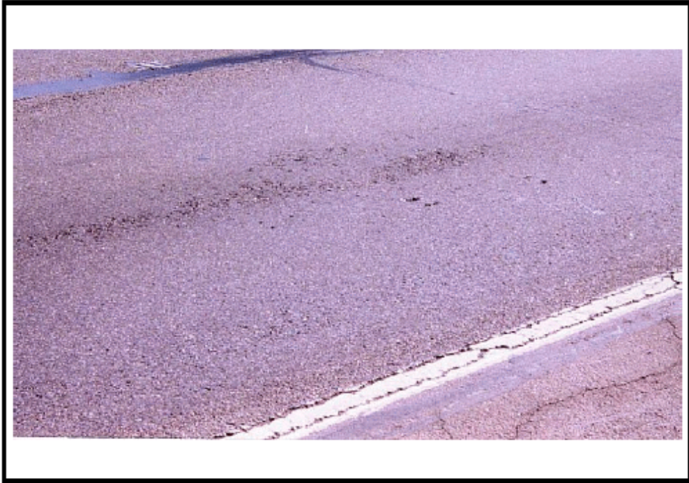
Photo A-1. Raveling in Flexible Pavement, Medium Severity
