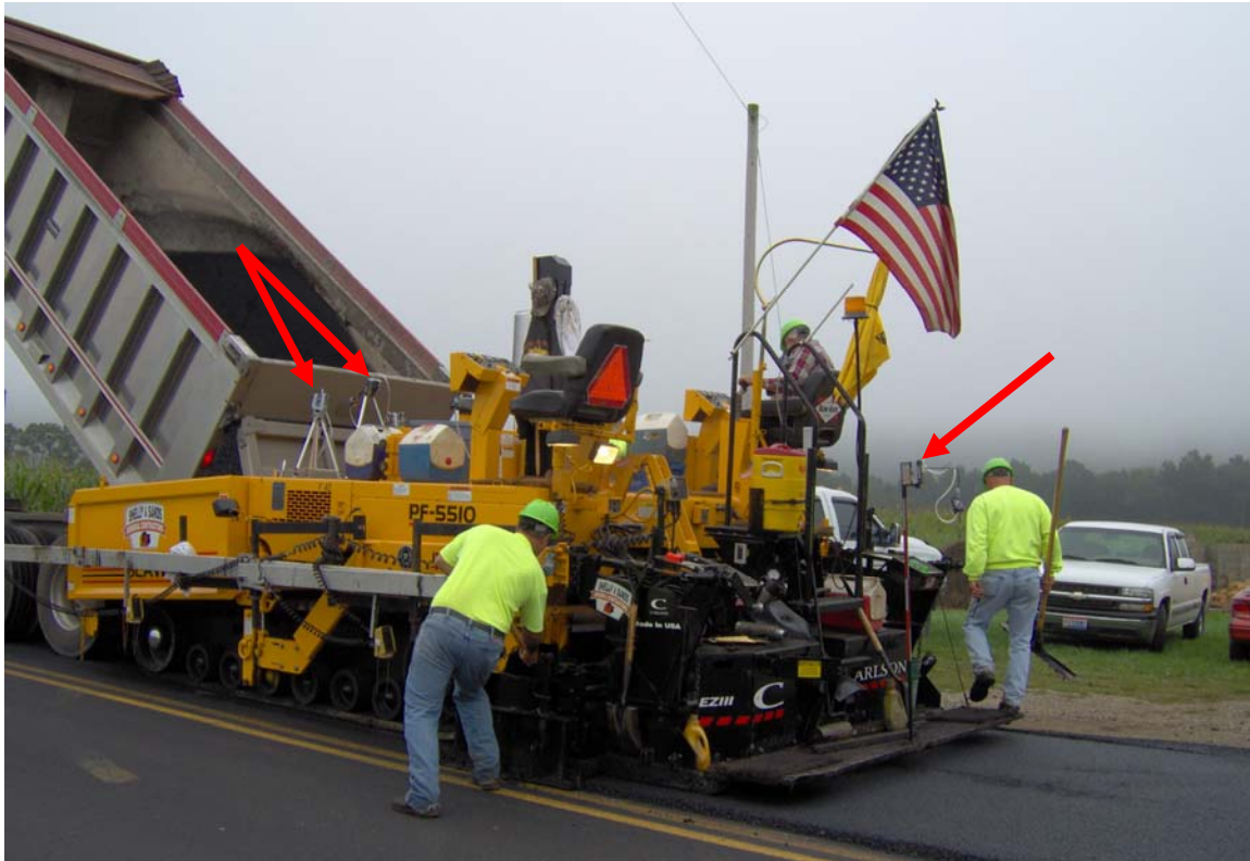
Figure 21. Photograph of the paving operation on SR541 showing monitoring equipment attached to paver, indicated with arrows. See Color Plate 8 in Appendix E.
