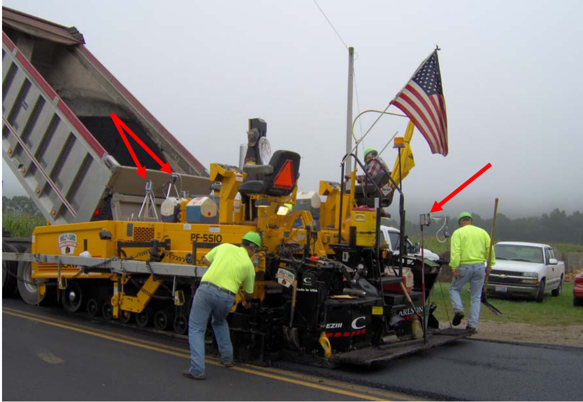
Color Plate 8. Photograph of the paving operation on SR541 showing monitoring equipment attached to paver, indicated with arrows. See Figure 21.
