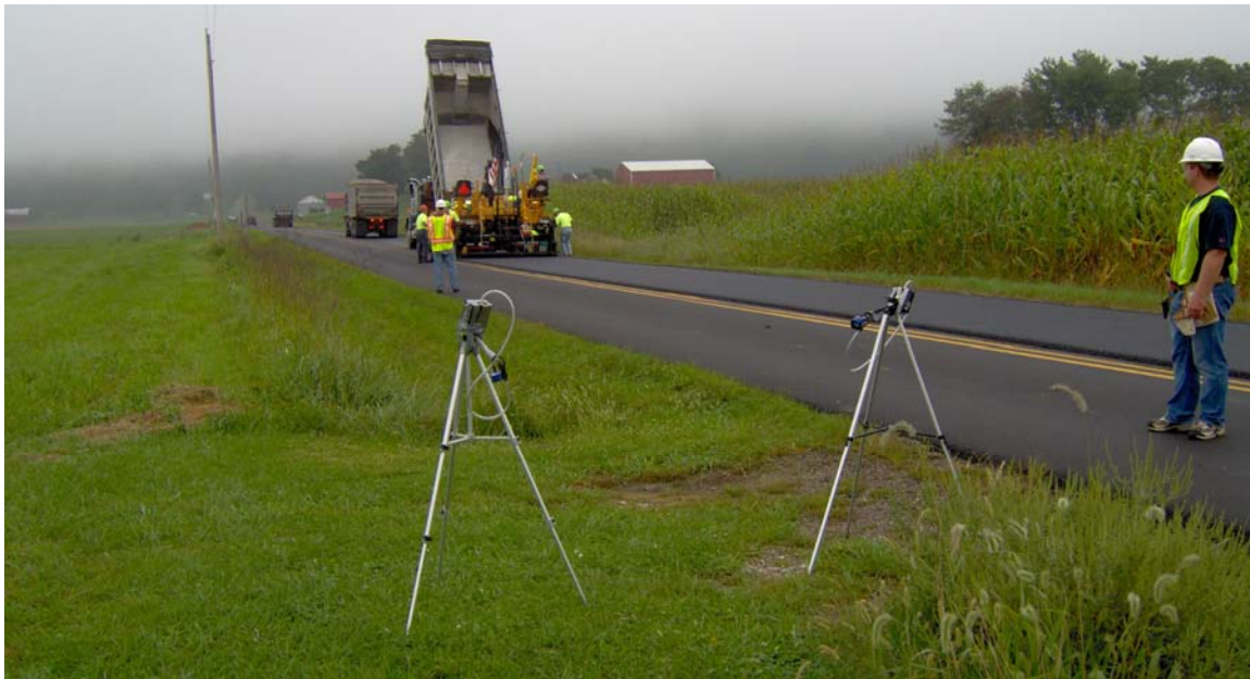
Figure 22. Photograph of paving operation on SR541, showing ambient air sampling equipment on tripods in foreground. The ambient air samplers are upwind of the paving. See Color Plate 9 in Appendix E.
