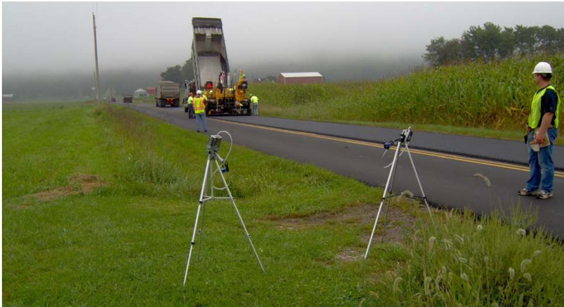
Color Plate 9. Photograph of paving operation on SR541, showing ambient air sampling equipment on tripods in foreground. The ambient air samplers are upwind of the paving. See Figure 22.
