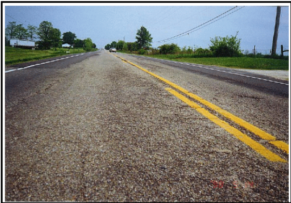
Photo A-2. Raveling in Flexible Pavement, High Severity
