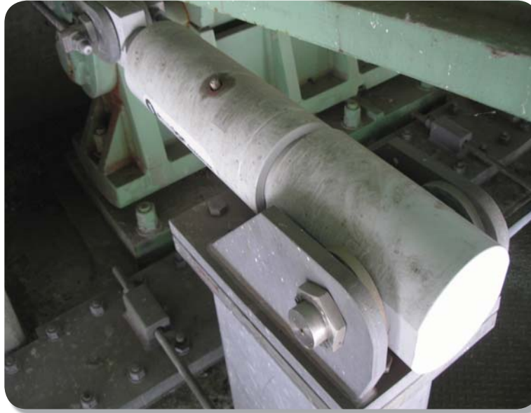
Figure 6.3 : Shock Transmission Units were Installed in Abernathy Bridge as Part of The Seismic Retrofit
