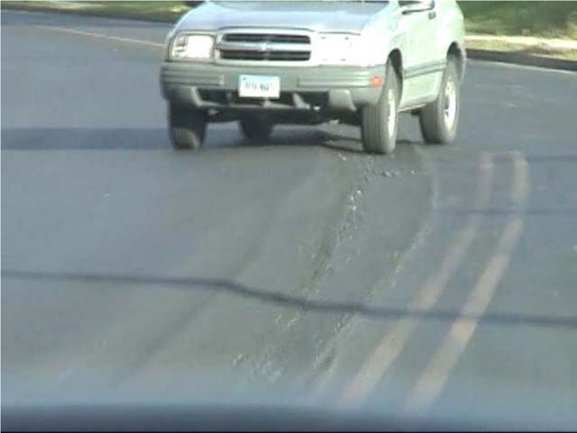
Figure 19 Traffic Traversing Open Joint
