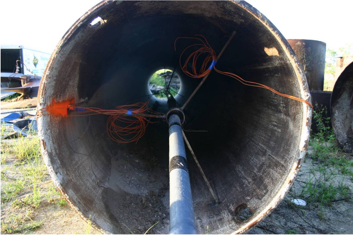
Figure 4-13. Thermocouples and access tube installed in center casing.
