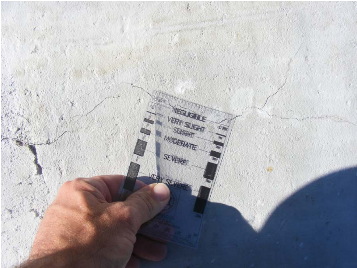
Figure 2-15. Although crack widths register as negligible, they run sporadically throughout wall.
