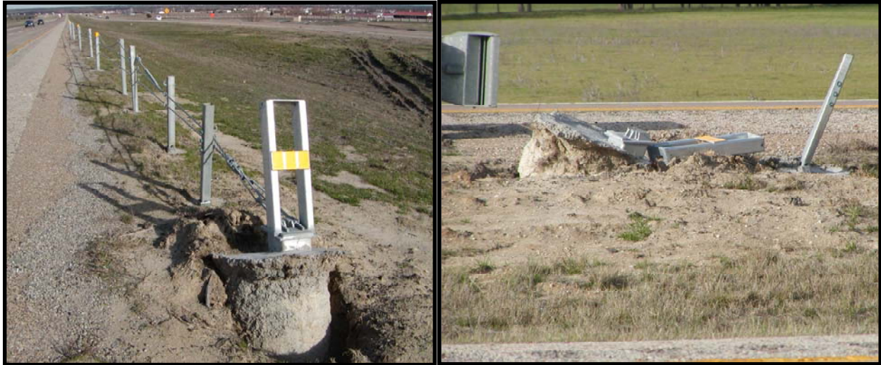
Figure 4-21. Anchor Failure on IH 20 Cable Barrier System in Kaufman County.
