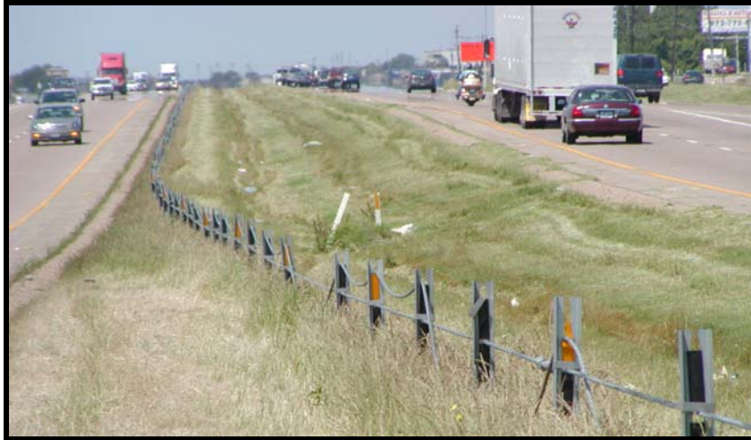
Figure 4-13. IH 30 in Rockwall – Top Cable Is Not Tensioned.
