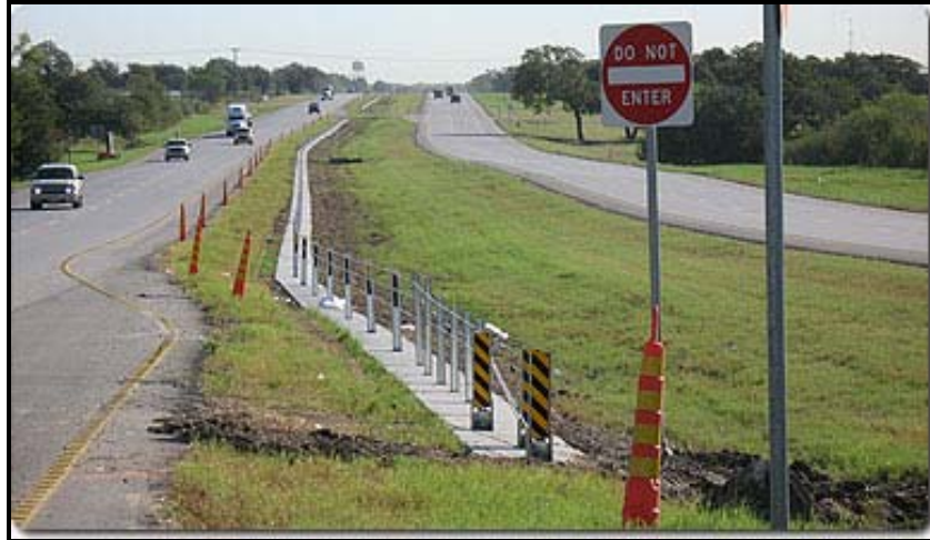
Figure 5-2. Cable Barrier System on State Highway 71 near Bastrop.
