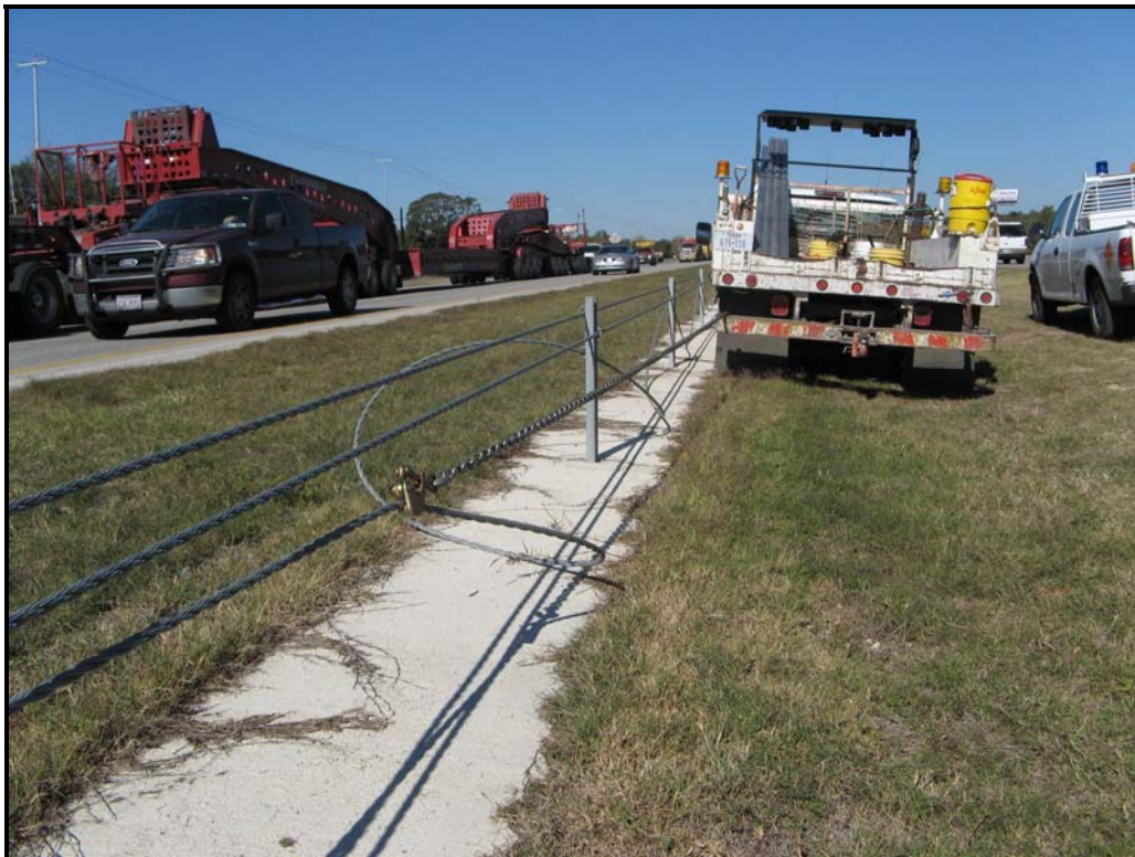
Figure 5-4. More Difficult Repair with Turnbuckle-Cable Separation on IH 10 in Boerne.
