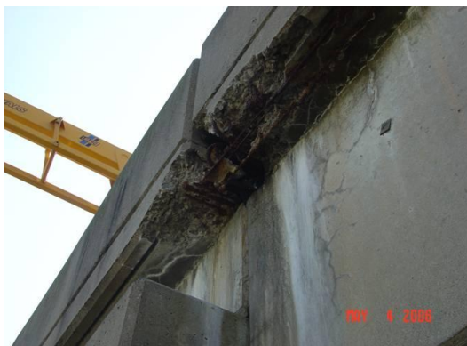
Sever spalling and reinforcement exposure on underside of parapet wall at Pier 3
