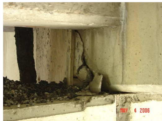
Cracking at the end of Beam 9, Span 1
