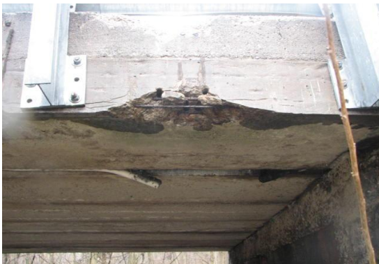
Spalling and exposed strands on exterior beam
