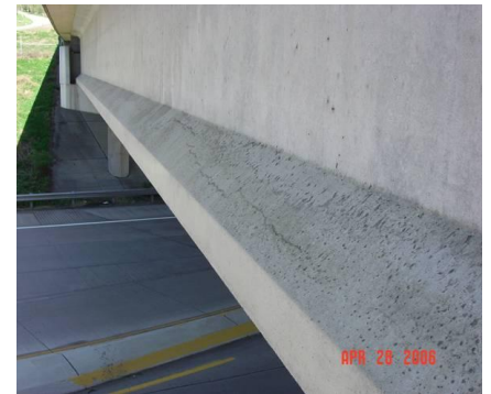
(c) longitudinal cracking resulting from impact.
