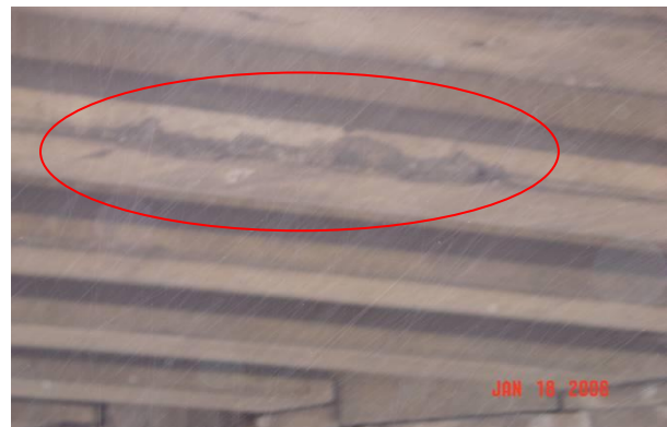
Span 3, Beam 6 – collision damage with spalling
