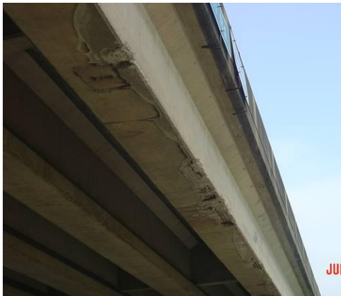
Collision damage on Beam 1, Span 2
