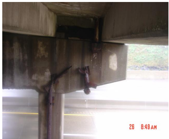
Poor downspout condition, typical for all on this bridge
