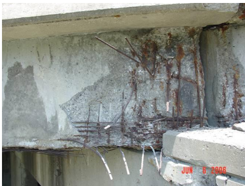
Beam 11 – exposed strands and reinforcing with heavy corrosion
