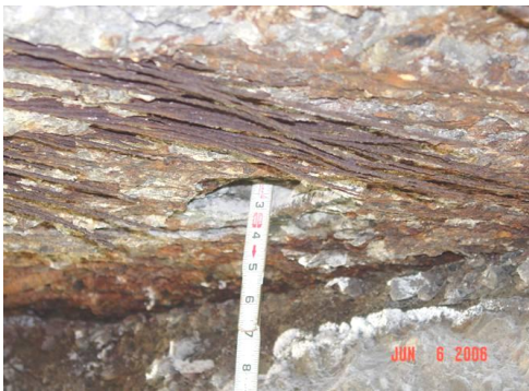
Beam 12 – Strand unraveled and 4" hole
