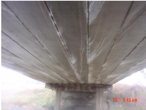
Heavy leakage between beams in Span 2
