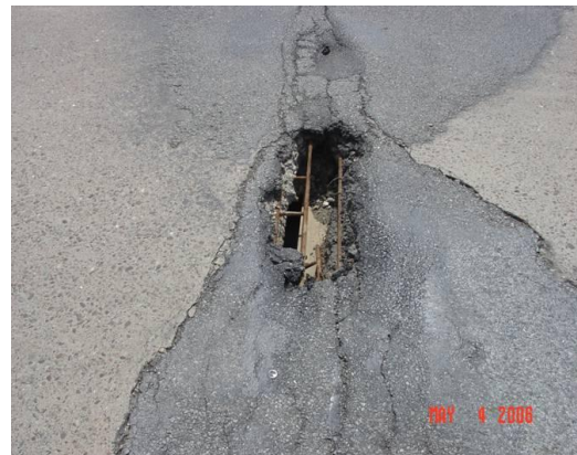
Hole through joint at Pier 3
