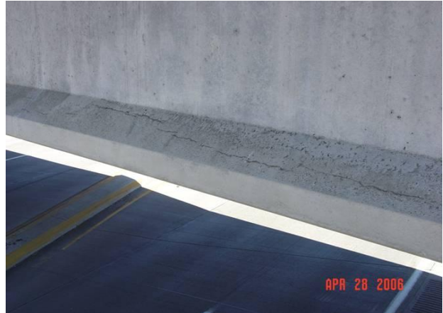
Longitudinal cracks in the bottom flange of B1
