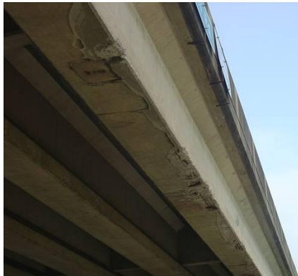
(a) damage to girder soffit.
