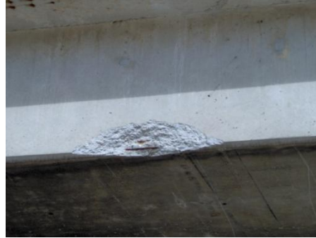
Close up of impact damage
