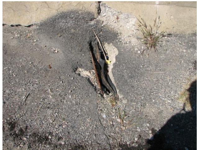
Hole in FLT paved joint
