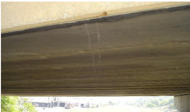
Scraping on underside of Span 4
