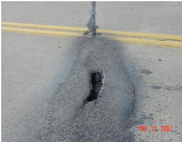
Hole in joint over pier
