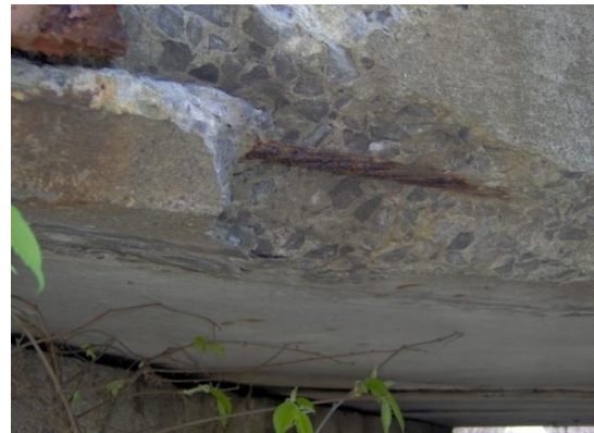
Continuation of spalling and strand exposure
