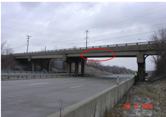
Location of collision damage on Beam 8
