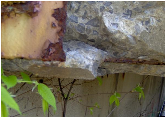
Spalling and strand exposure at beam end
