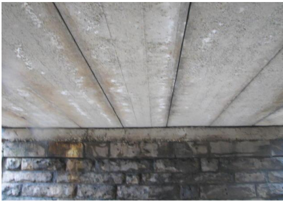
Underside of bridge with moisture and staining in between beams
