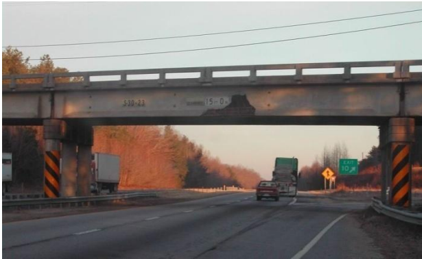
Figure 1.1 Loss of section of AASHTO girder due to vehicle impact (Harries; not taken in PA).
