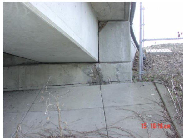
Spalling under B1 at NAB
