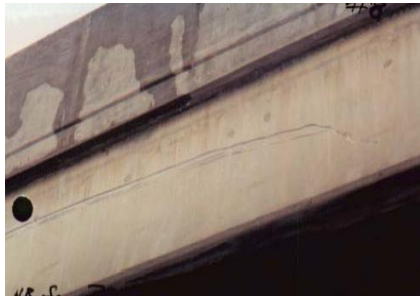
(b) typical impact damage pattern (PennDOT).
