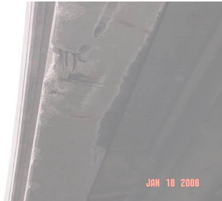
Span 3, Beam 8 – collision damage with exposed and severed strands
