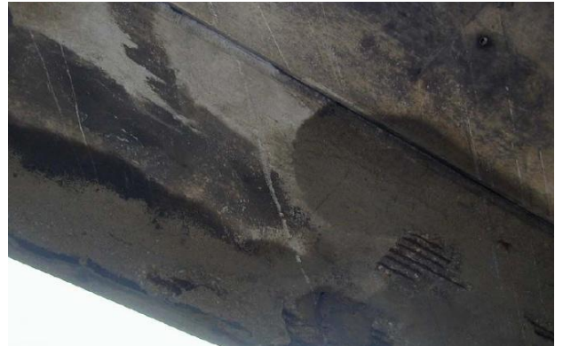
Figure 1.2 'Scraping' due to minor vehicle impact (Lake View Drive Bridge prior to collapse; PennDOT and Harries 2006).
