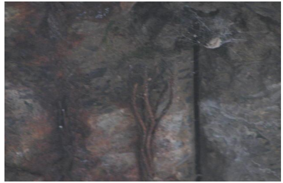
Beam 8 - Close up of broken strands
