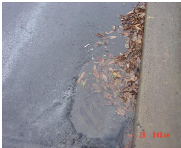
Clogged inlet of Span 1
