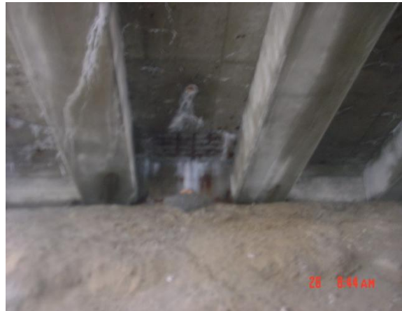
Exposed rebar in the underside of the deck between beams 4 and 5
