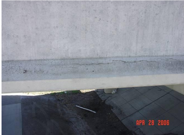
Longitudinal cracks in the bottom flange of B1
