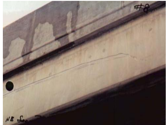
Longitudinal crack from impact damage
