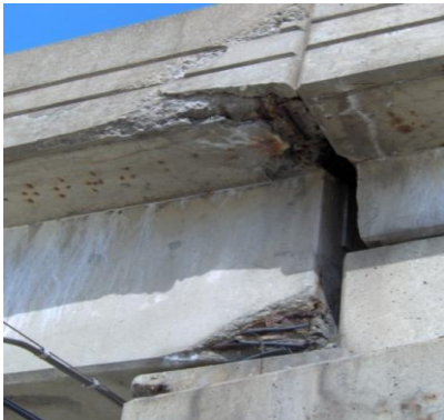
Beam end spall and parapet spalling
