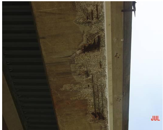
4 broken strands in Beam 1 at location of collision damage
