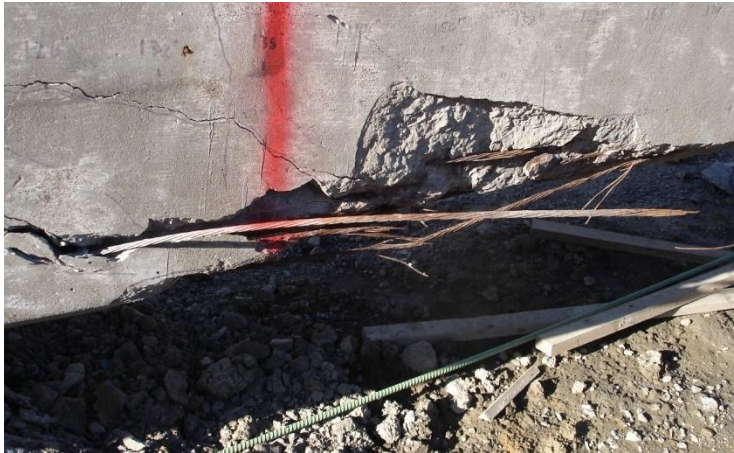
Figure 7.1 Strand following induced failure of Lake View Drive girder. The 3/8" strand is entirely lost to corrosion at right of image. At left of image, where it was pulled out of sound concrete (left of red paint line) the strand is 'bright steel' with no section loss. (photo: Harries)
