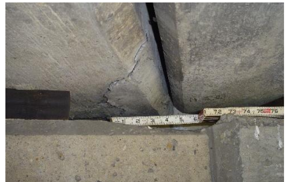
Bottom corner of beam S7, cracked and delaminated at pier
