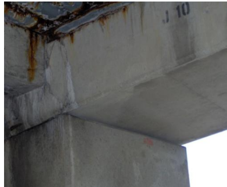
Efflorescence and cracking at beam end
