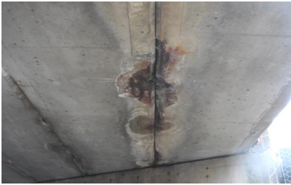
Beam 8 – Spalling, exposed strands and rust on side
