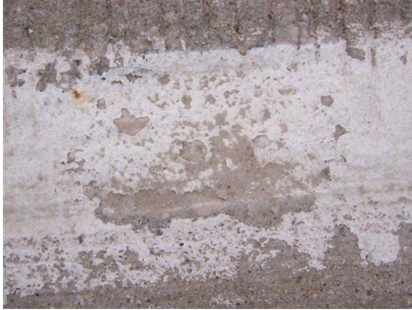
Figure 5-14. Peeling paint chips on flat area
