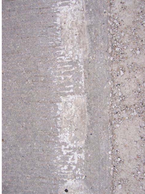
Figure 5-18. Another portion of P-53 showing less wear in the rumble stripe than in the flat area (taken spring 2009)
