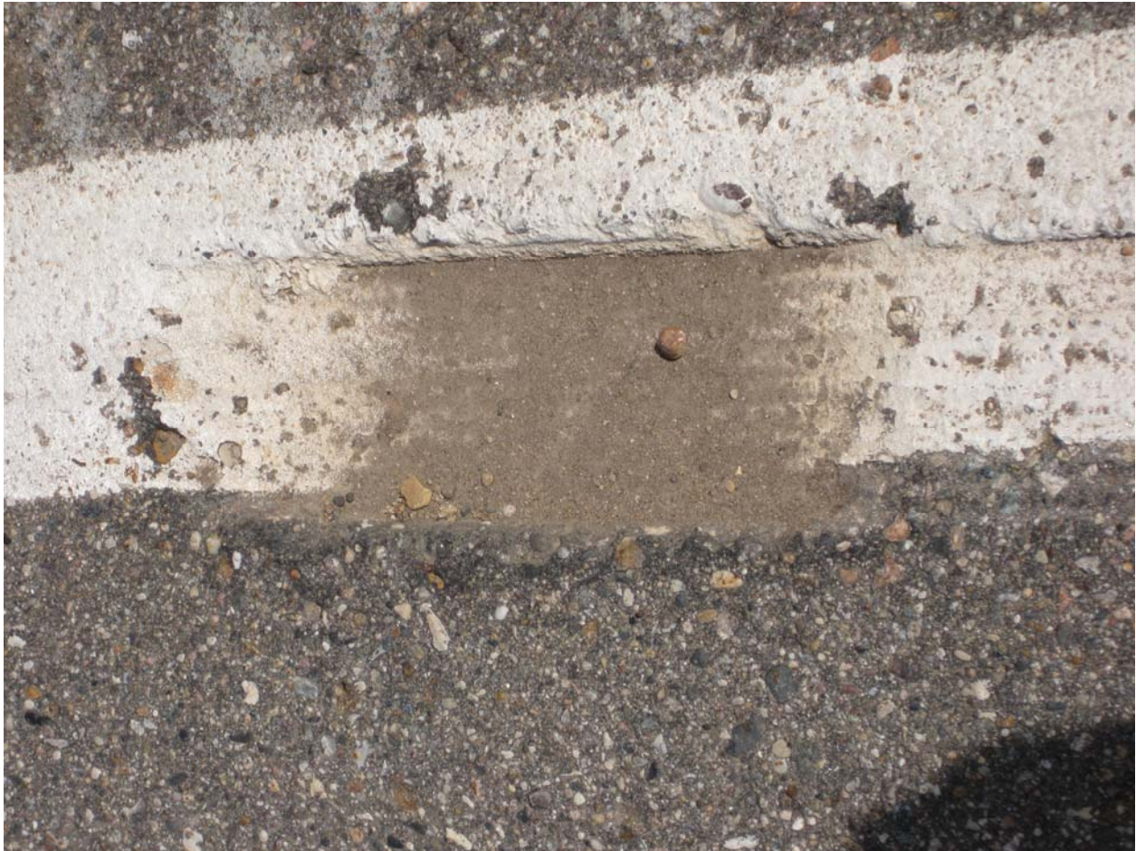
Figure 6-1. Rumble stripes on B-30 filled with debris
