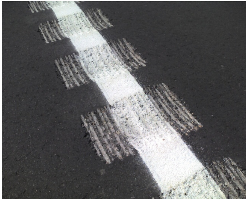
Figure 1-1. Four-inch edge line rumble stripe placement on a rural highway in Iowa
