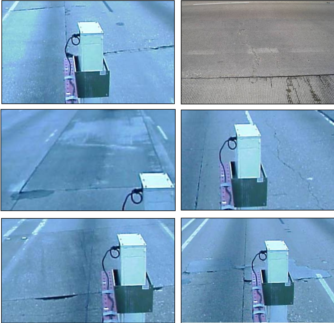
Figure 27. Surface Condition of Sampled Section on IH 635.
