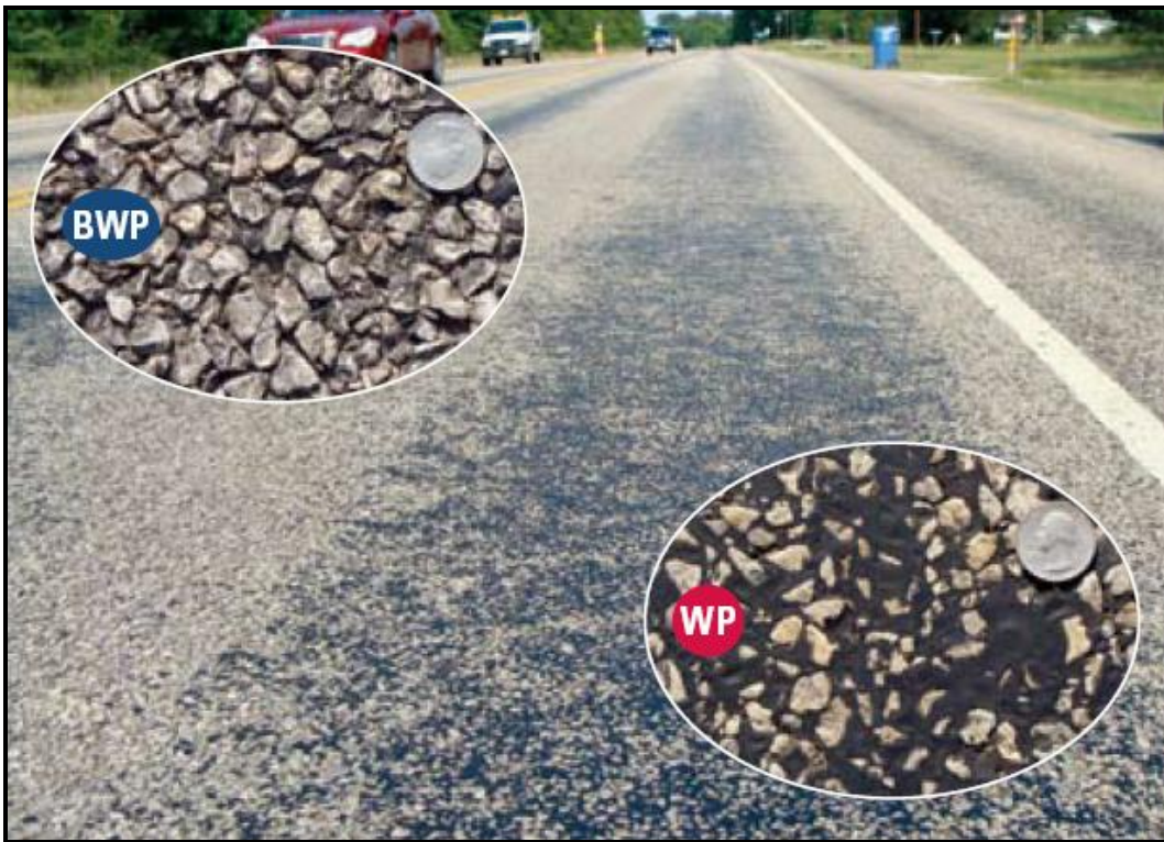
Figure 18. Moderate to Severe Flushing of Grade 3 Seal Coat.
