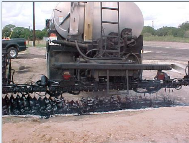
Figure 3 – Blowing Out Spray Bar
