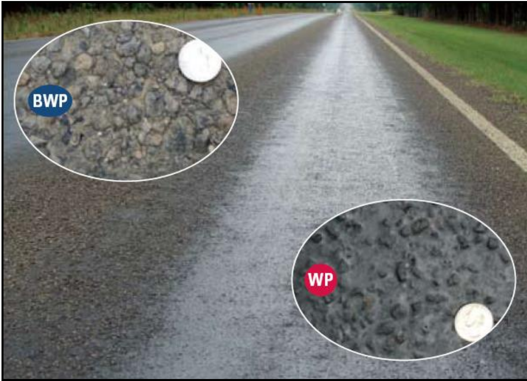
Figure 17. Severe Flushing of Grade 3 Seal Coat.
