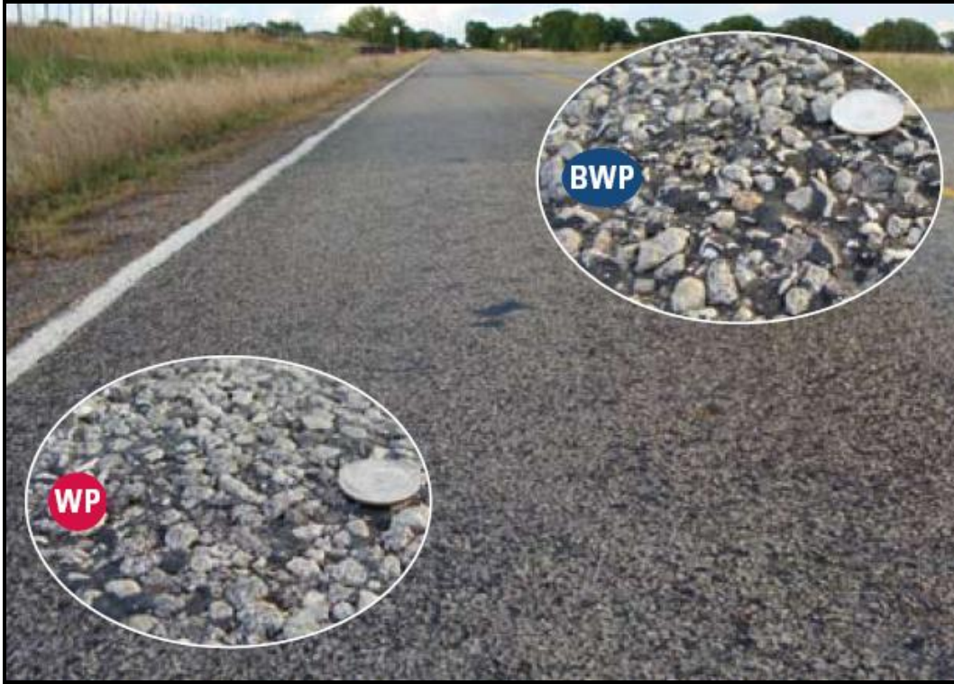
Figure 21. Mild Flushing of Grade 3 Seal Coat.
