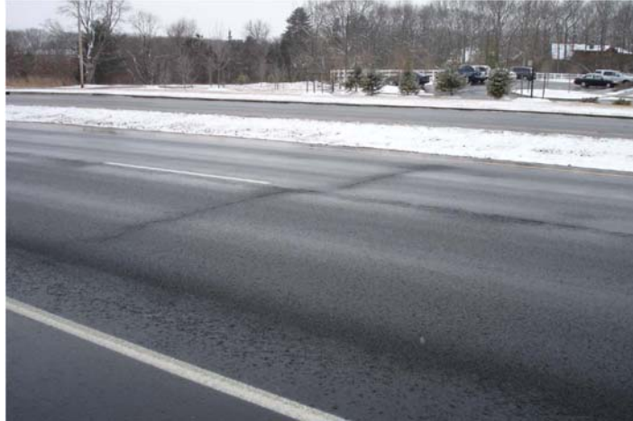
Figure 4. Reflection Cracking in Route 34 NB, New Jersey (21).
