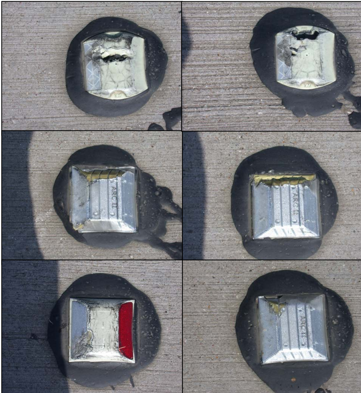
Figure 81. Typical RRPM Damage on Concrete Pavement in Rural Laredo.
