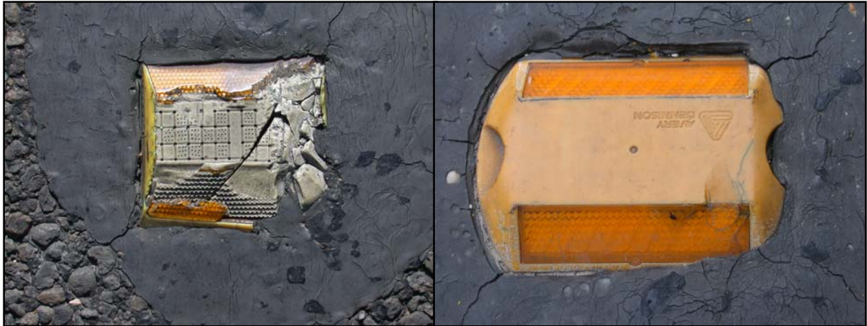
Figure 87. Typical RRPM Damage on Seal Coat Pavement in Lufkin (Continued).
