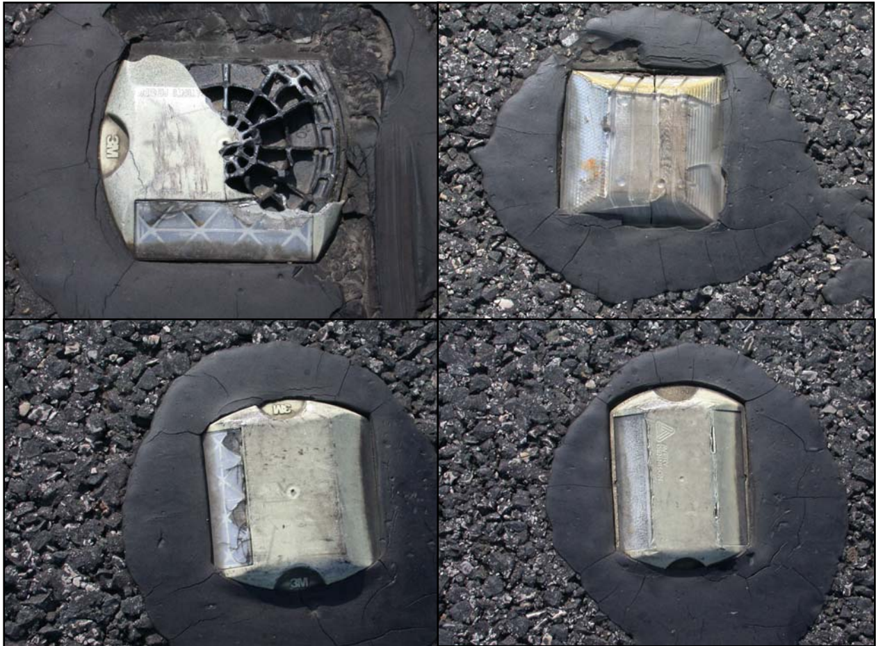
Figure 78. Typical RRPM Damage on Asphalt Pavement in Rural Laredo (Continued).
