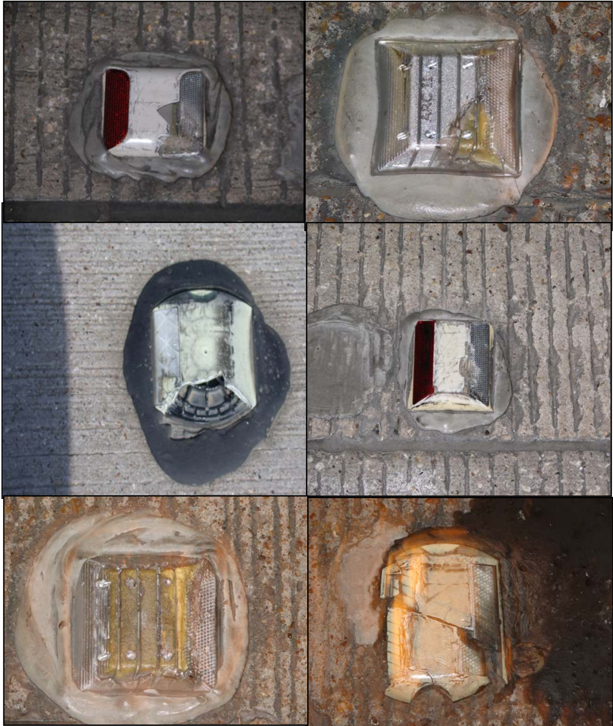
Figure 84. Typical RRPM Damage on Concrete Pavement in Houston.
