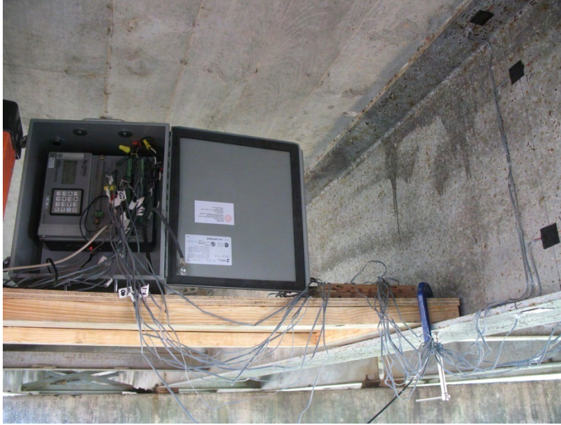
Figure 4.5: CR 500 data logger used for field tests
