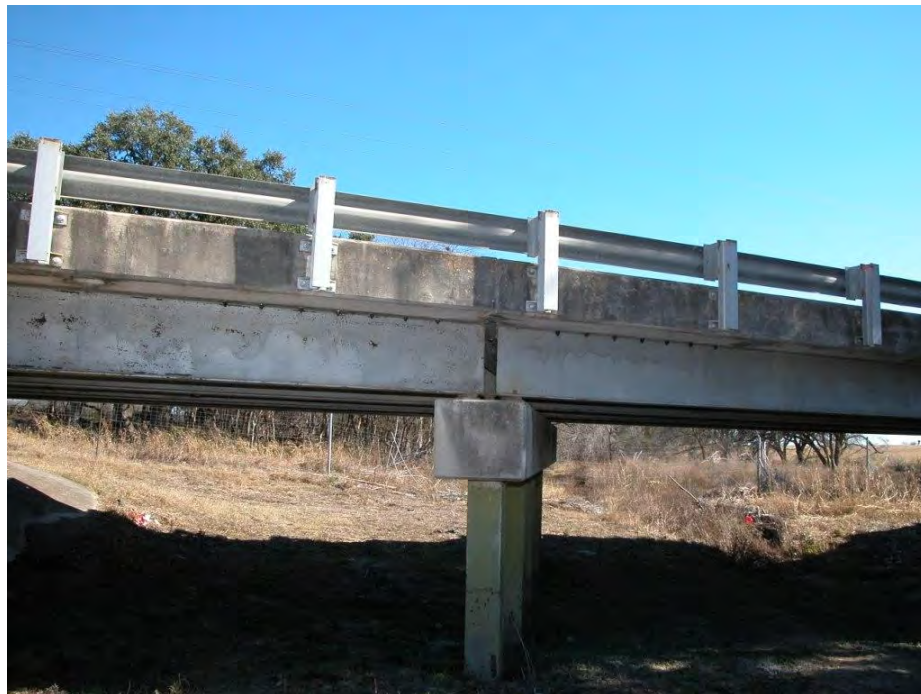
Figure 3.19: Post-installed shear connectors in exterior girders of north span (on left) and center span of Hondo Bridge (DBLNB in north span; HTFGB in center span)
