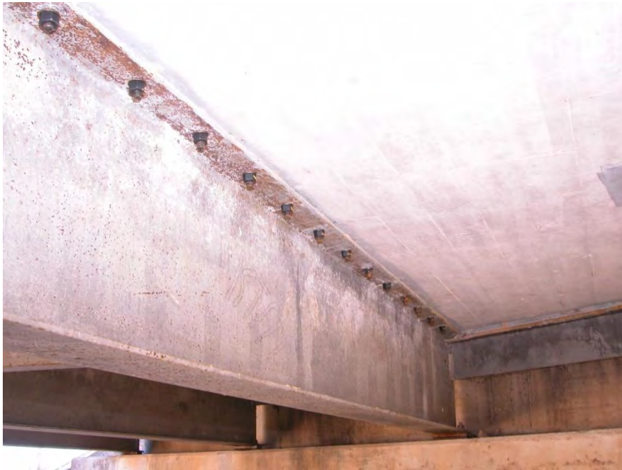
Figure 3.17: Post-installed shear connectors (HASAA) in an interior girder in south span of Hondo Bridge
