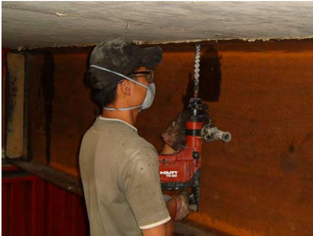
Figure B.12: Drilling into the concrete slab using a rotary hammer drill
