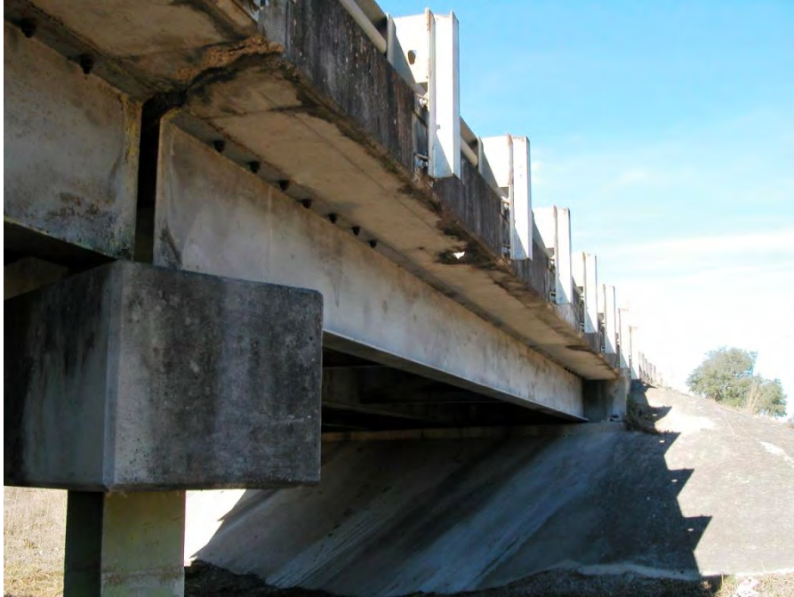
Figure 3.18: Post-installed shear connectors (DBLNB) in an exterior girder in north span of Hondo Bridge
