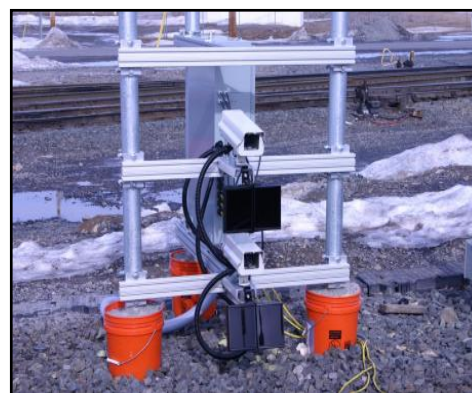
Figure 3: The BPMS module at the Selkirk installation
