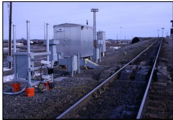
Figure 10: WISE at the CSX Selkirk location
