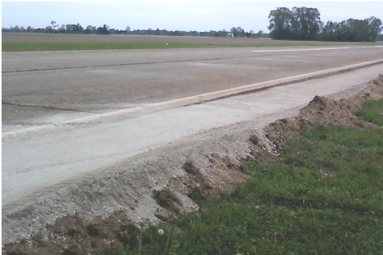
Figure 6. Photograph. The beginning of the gravel shoulder was flush with the runway, as is visible at the left. A ramp leads to the four-inch vertical edge.
