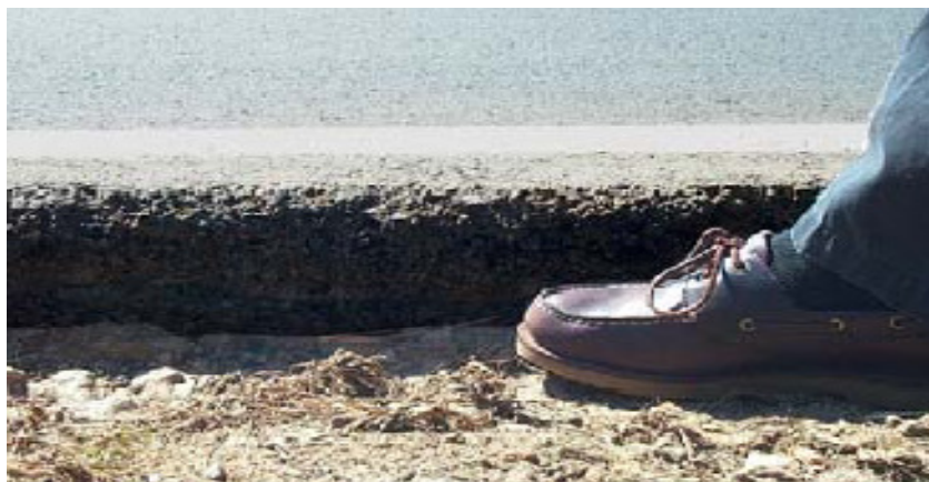
Figure 4. Photograph. A vertical pavement edge with an unusually high drop-off.
