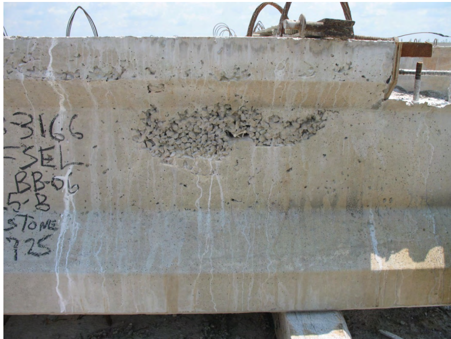
Figure 5-17 Sample of honeycombing in box beam BB-06
