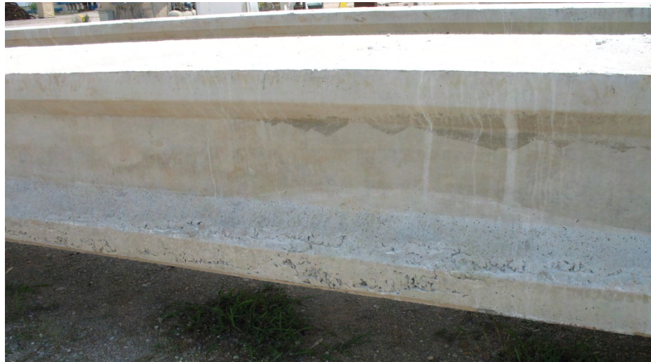
Figure 5-18 Sample of honeycombing in box beam BB-07
