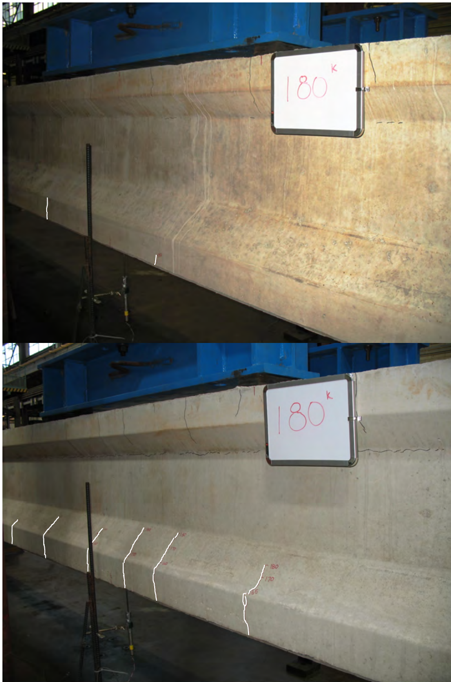
Figure 5-29 Visually observed cracks of beam BB-01 and BB-06 respectively at an applied load of 180-kips
