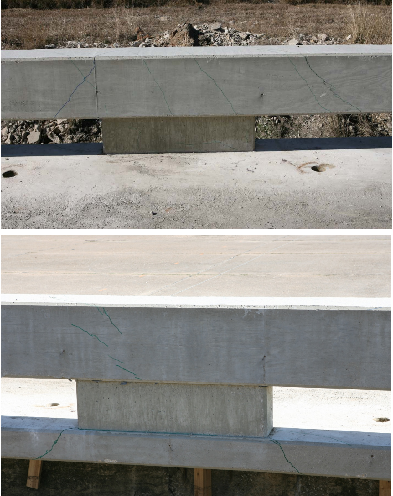
Figure 25. Installation after Test 452109-B4.
