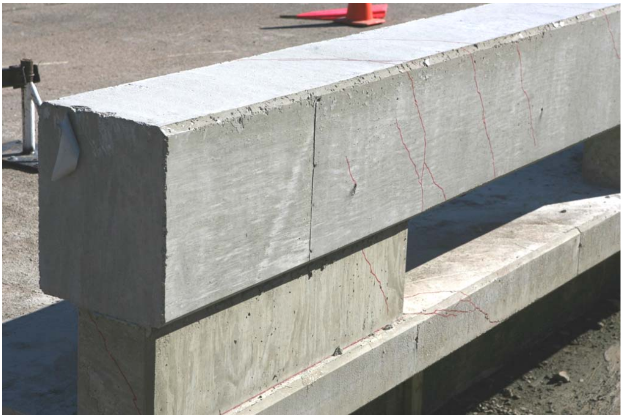
Figure 17. Installation after Test 452109-B2.
