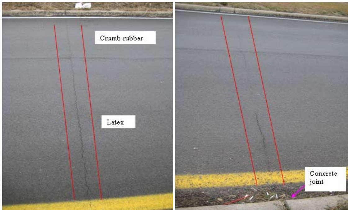
Figure 27b. Reflected Transverse Cracking through Concrete Joints (Ramp R1).
