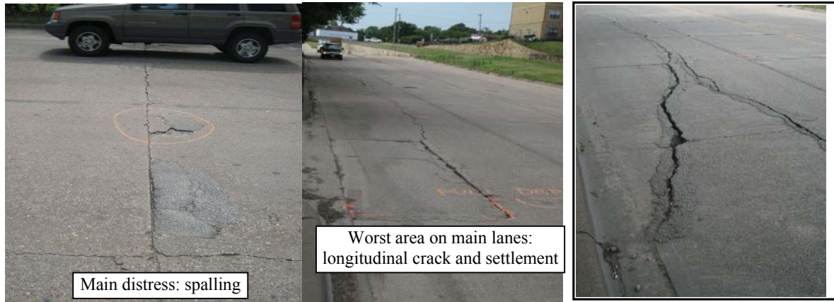
Figure 21. Observed Distresses on the Main Traffic Lanes, Pumphrey Drive, FTW.
