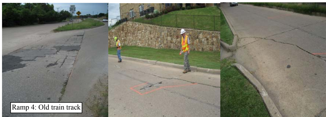
Figure 22. Observed Distresses on the Ramps, Pumphrey Drive, FTW.
