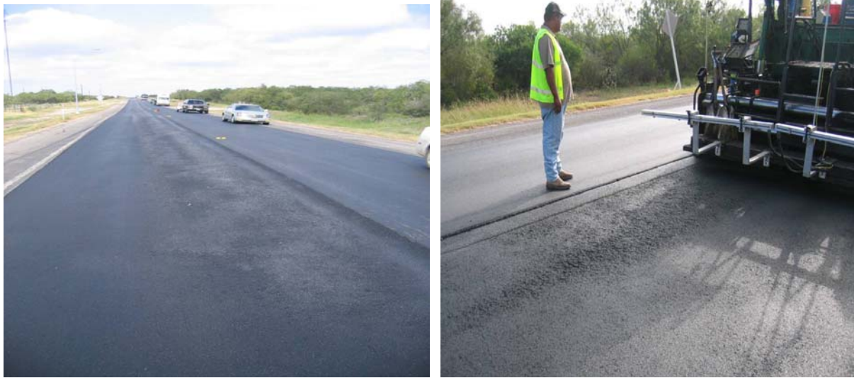
Figure 40. Placement Problems with the CAM on US 90.
