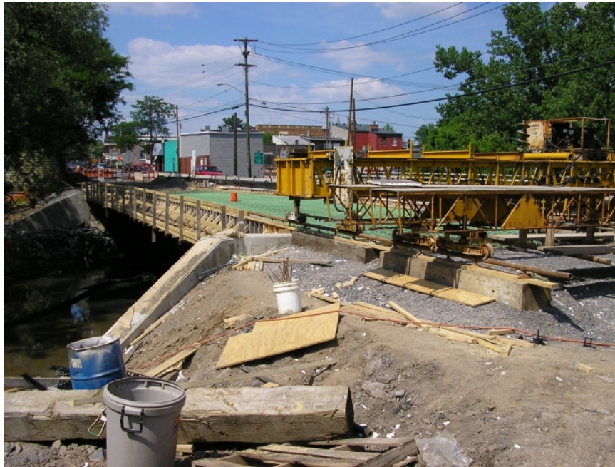
Figure 20: Photograph of the formwork and rebars, prior to casting concrete for the bridge deck in Region 3 (Courtesy Jonathan Kunin, NYSDOT).
