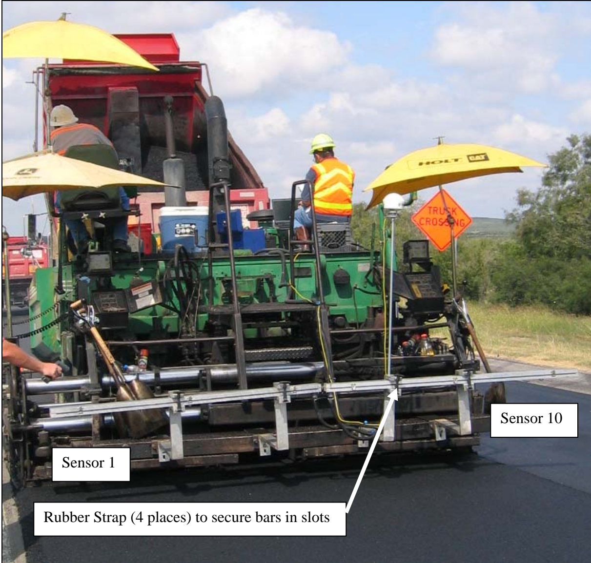
Figure 5. IR Bar Mounts with IR Bars Installed.
