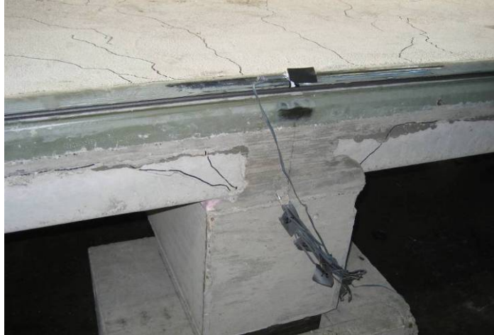
Figure 5.11: Photograph of Specimen N0P1 after Punching Shear Failure
