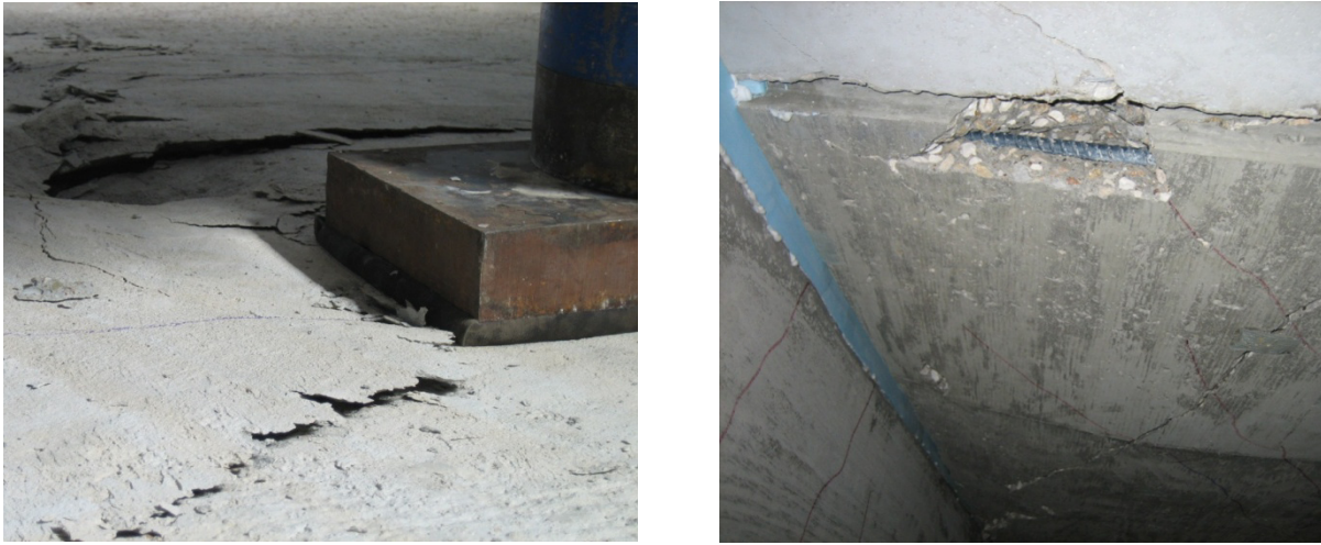
Figure 6.13: Failure of Specimen 6 under Loading at Joint Between Panels
