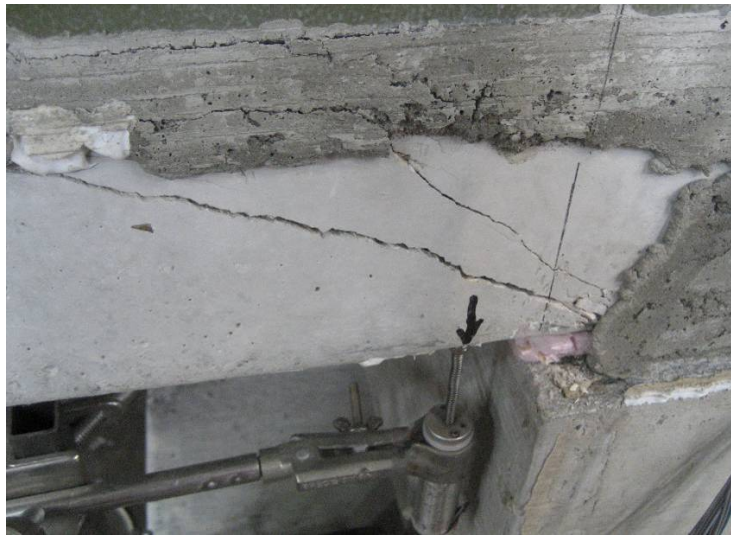
Figure 5.14: Photograph of Specimen 4 after Shear Failure near Center Support
