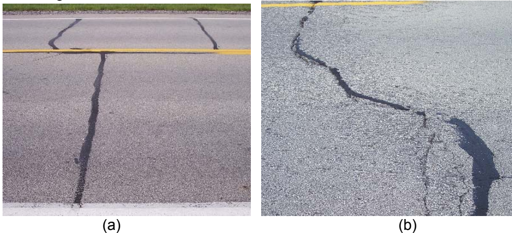
Figure A.18.3 Severity of sealed crack: (a) low and (b) medium (up) to high (down) level.
