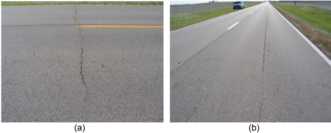
Figure A.15.3. (a) Unsealed transverse cracks and (b) unsealed longitudinal cracks.
