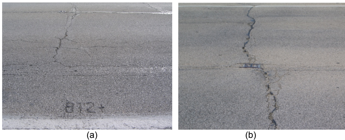
Figure A.12.3. Medium-severity-level transverse crack: (a) unsealed and (b) sealed one.
