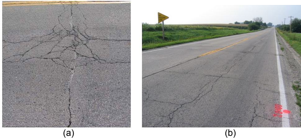
Figure A.6.3. (a) High-severity-level cracking and (b) block cracking.
