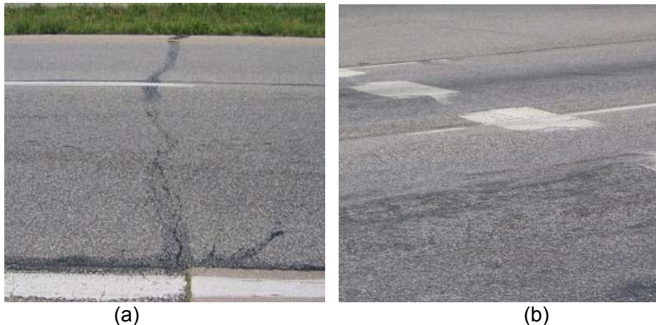
Figure A.22.3. (a) Medium-severity-level transverse crack and (b) bleeding and rutting.
