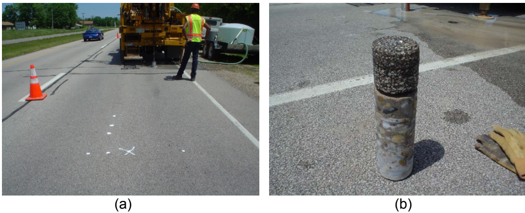
(a) (b) Figure 4 Field coring work: (a) Coring locations (b) Coring samples.
