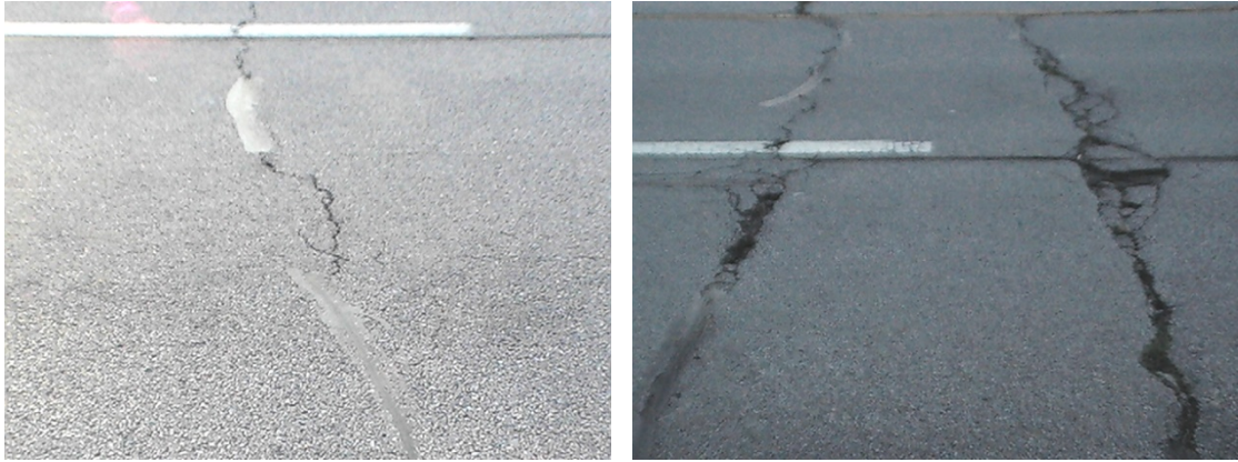
(a) (b) Figure A.9.3 Transverse cracking: (a) Medium and (b) High severity
