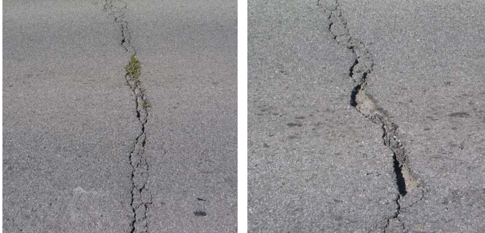
Figure A.24.3. Highly deteriorated double reflective cracks
