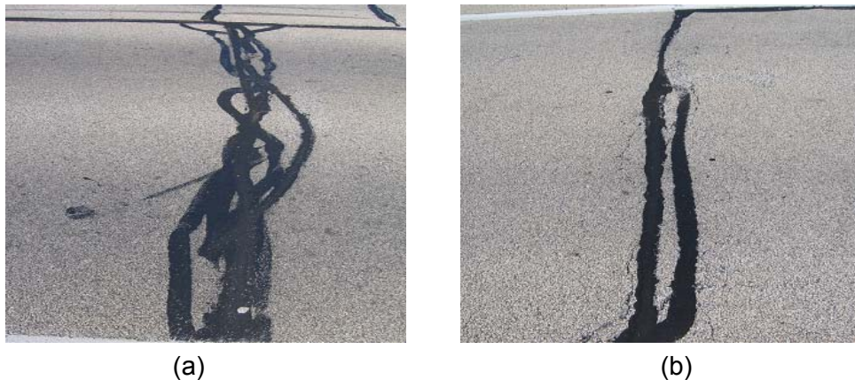
Figure A.23.2. Sealed transverse reflective cracking: (a) low-level and (b) medium-level.
