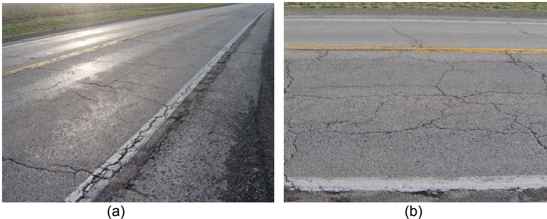
Figure A.8.3. (a) Unsealed longitudinal and transverse cracking and (b) block cracking.
