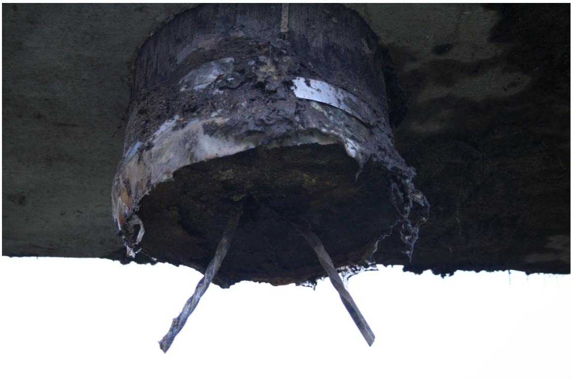
Figure A-11. Failed post connection.
