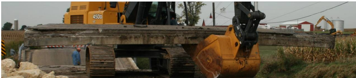
Figure A-4. Extracted deck beam.
