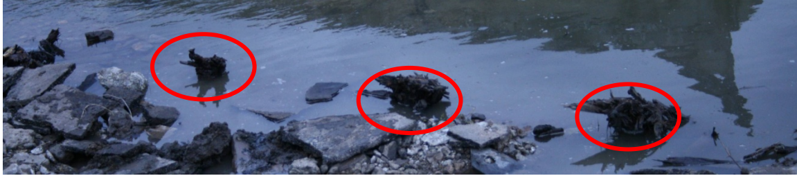
Figure A-12. Piles remaining in riverbed.
