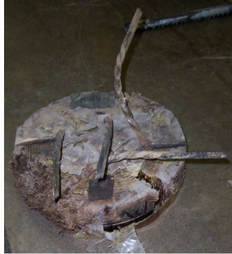
Figure 4. Damaged "post" connection.
