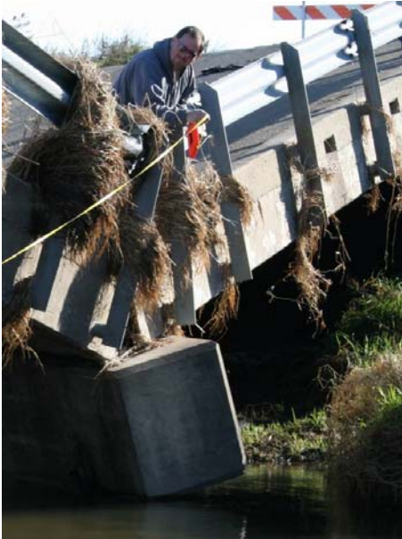
Figure A-5. Collapsed bent 3 pile cap.
