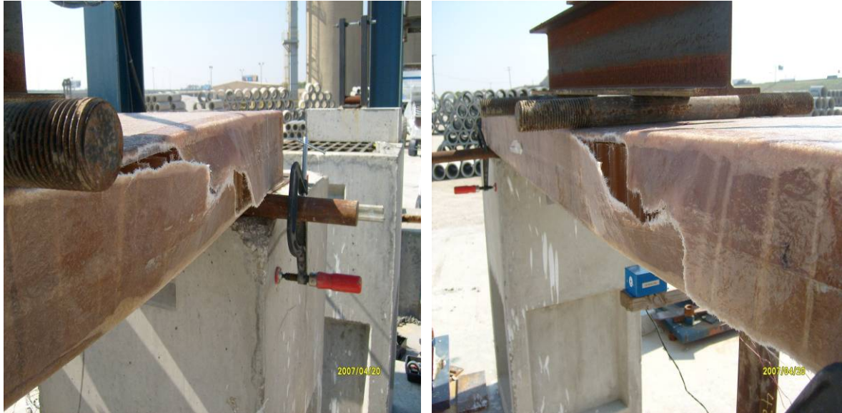
Figure 4.14: Fiber Deck with Transverse Ribs at the Point of Failure
