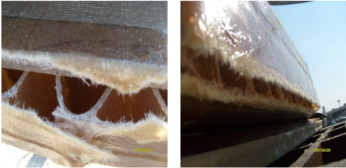
Figure 4.10: Fiber Deck with Longitudinal Ribs at the Point of Failure
