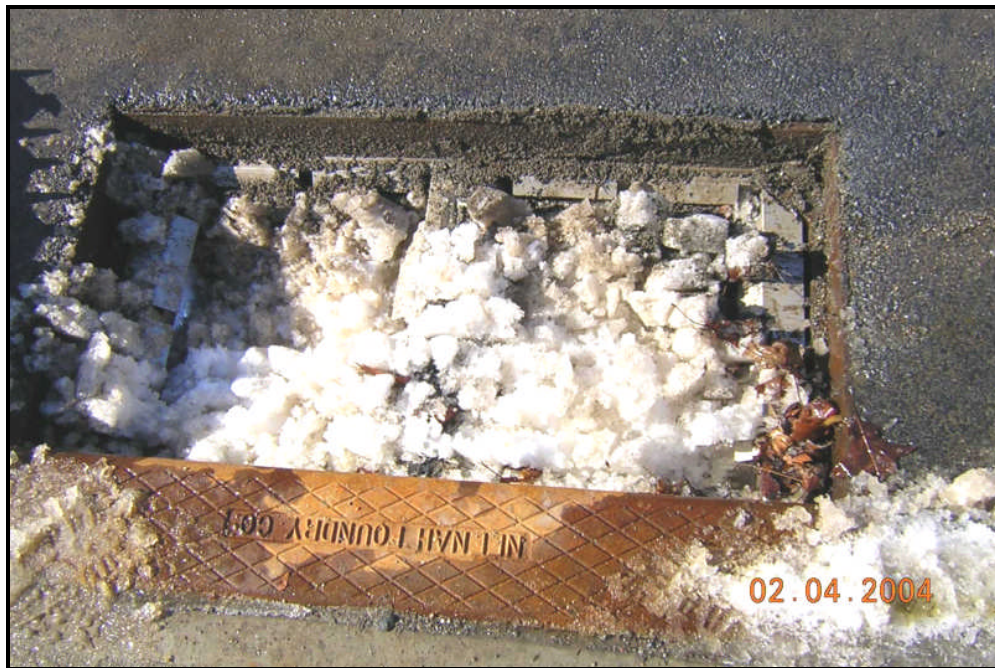
Figure 45: Snow covering the FloGard ® +PLUS Filter
