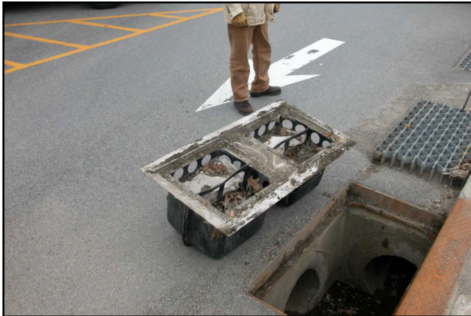
Figure 49: Catch basin where the Hydro Kleen® was installed
