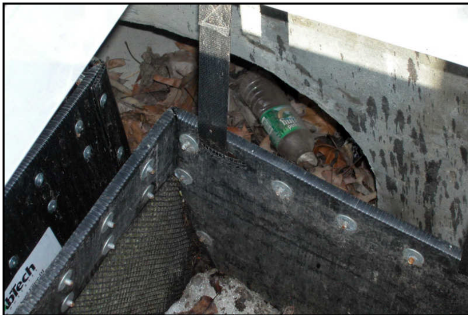
Figure 53: The Ultra-Urban® obstructed the drainage pipe
