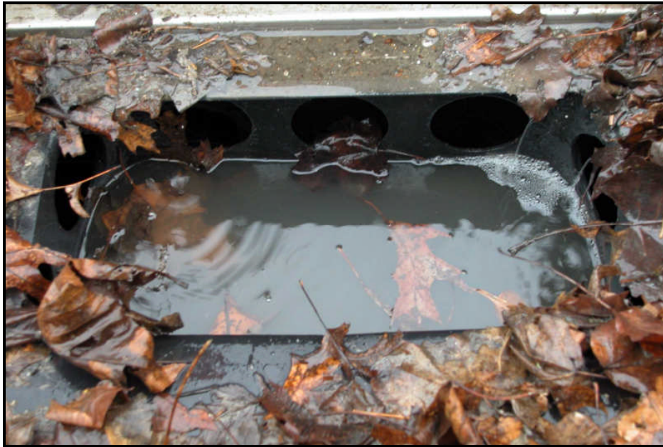
Figure 48: Hydro-Kleen™, the overflow by-pass is close to the standing water level
