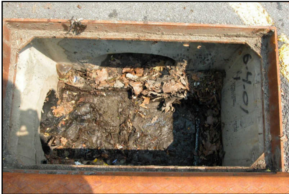
Figure 54: Catch basin where the Ultra-Urban ® Filter was installed
