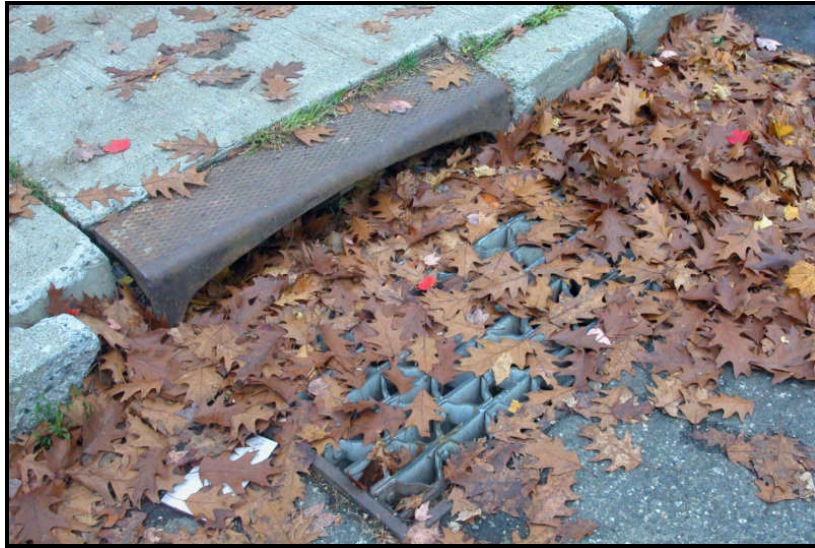
Figure 38: Catch basin covered with leaves during the fall season
