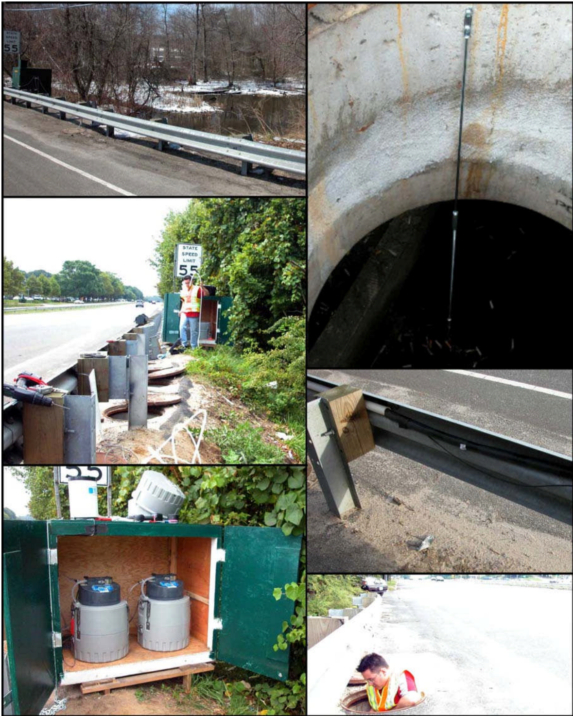
Figure 68: V2b1™ – Sampling system installation
