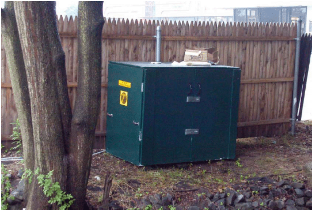
Figure 58: Storage box in Bayshore – Vortechs® System
