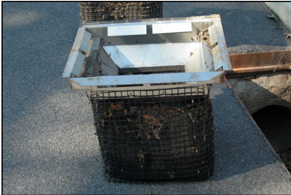
Figure 46: FloGard ® +PLUS is deep and can obstruct connecting drainage piping
