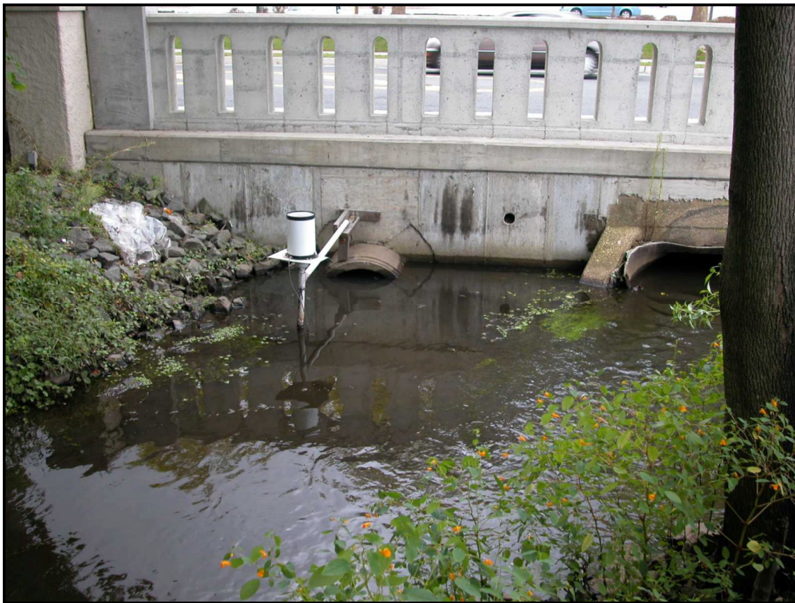
Figure 66: Vortechs® Sampling System – Rain Gauge
