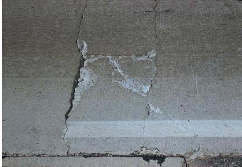
Figure 2.1: Typical CRCP punchout distress (Source: FHWA HRT-04-122, 2005, Figure 64)
