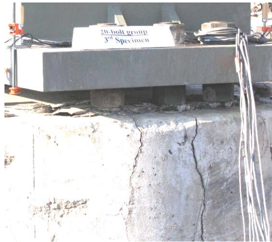
Figure 5.7 Contact of Nuts with Top Surface of Drilled Shaft
