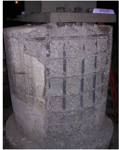
(c) After failure
