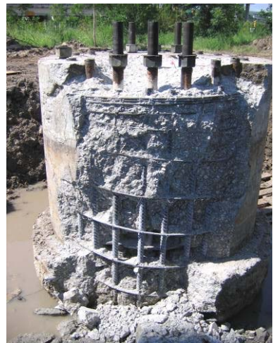
(c) After failure
