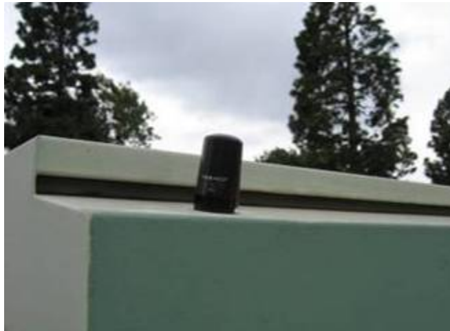
Figure 4-16: Typical WLAN Client Antenna Installation
