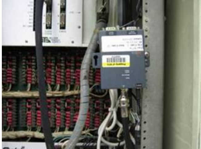
Figure 4-15: Typical WLAN Client Intersection Cabinet Installation
