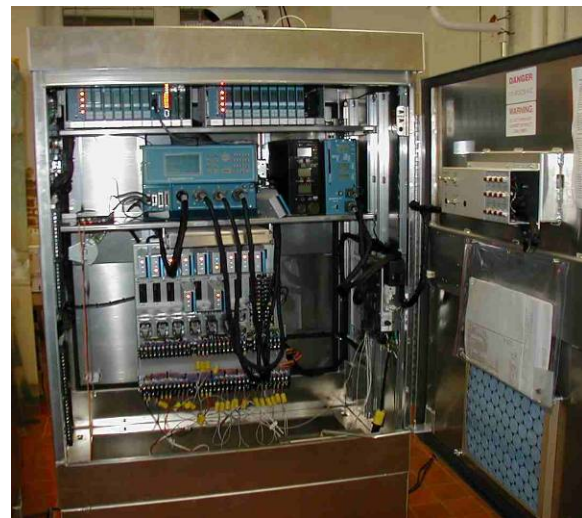
The traffic controller cabinet shown above includes a NEMA Econolite ASC/2 controller. Photo Credit: Peter Koonce
