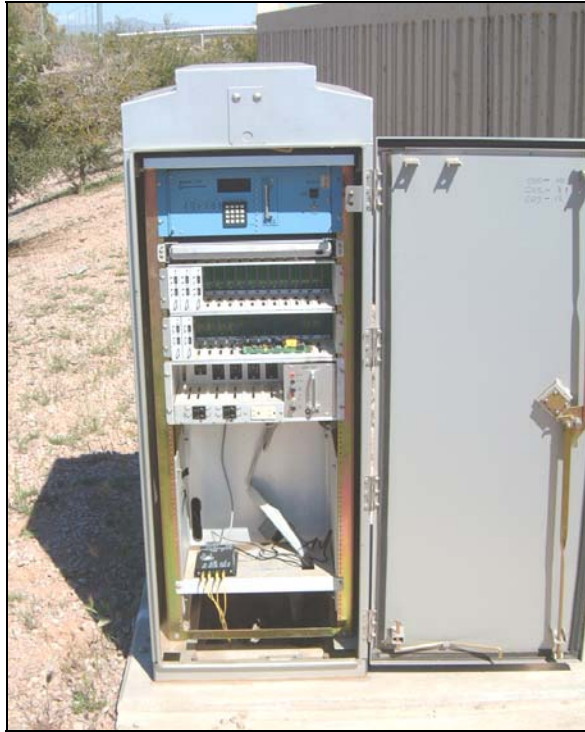
Figure 2: FMS Cabinet with Inductive Loop Equipment
