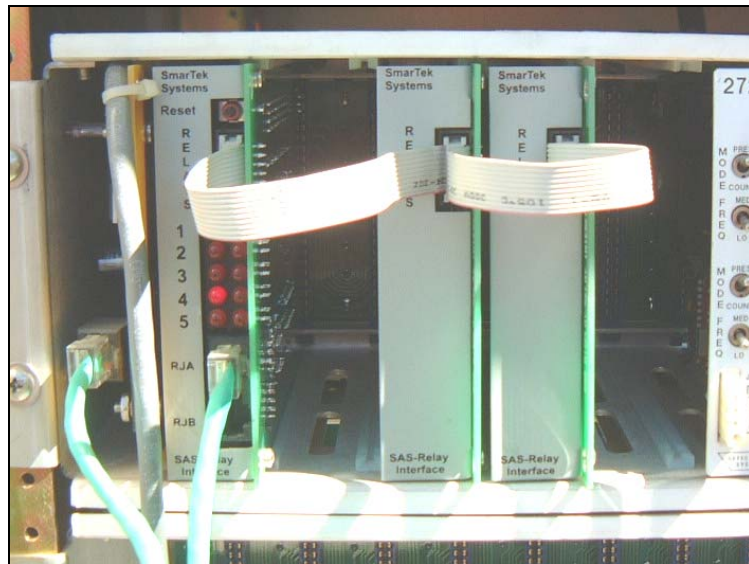
Figure 3: SmarTek SAS-1 Contact-closure Cards
