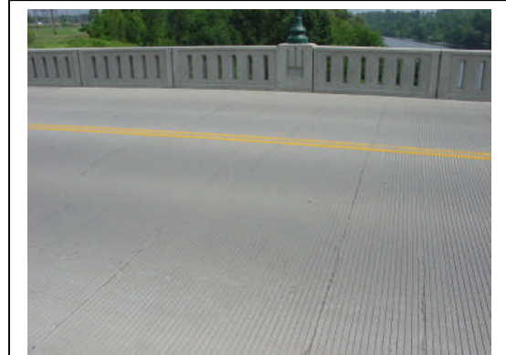
Figure 5 - Cracking in BIN 3221420, Alcoa Road over Grasse River constructed in 2002.
