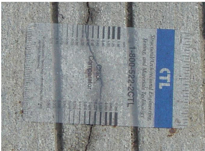
Figure 15 - Close up of one of many cracks in BIN 3221420 - Alcoa Road over Grasse River
