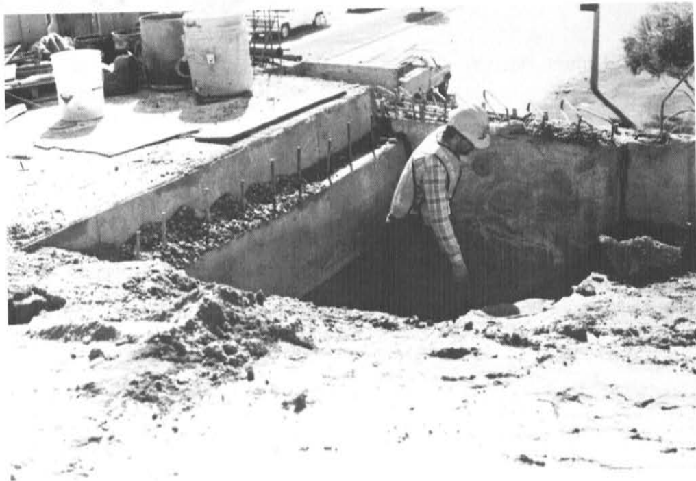
Figure No. 32 The Depression Formed at the Top of the Wall Due to the Seeping of the Backfill Thru the Wall's Bottom
