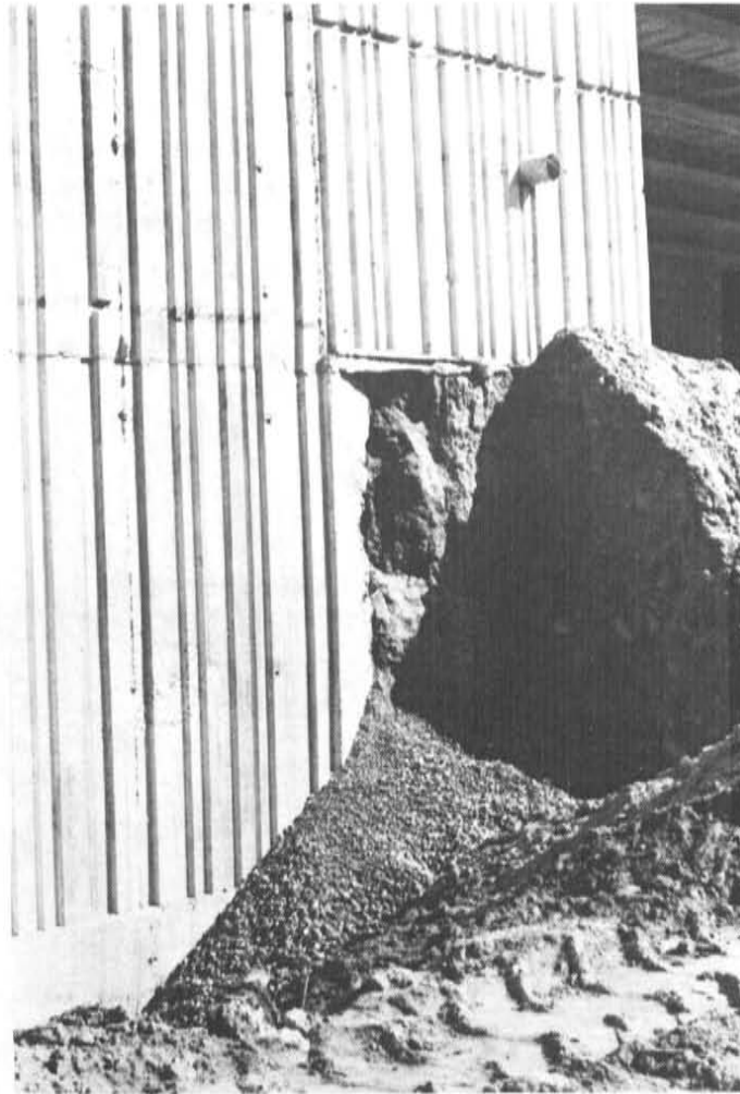
Figure No. 31 The Backfill Material After Seeping Thru the Crevices
