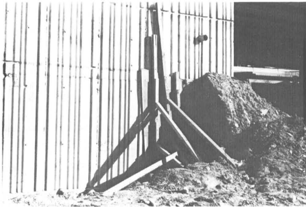
Figure No. 33 Corrective Measure Taken for the Crevices at the Bridge Abutment
