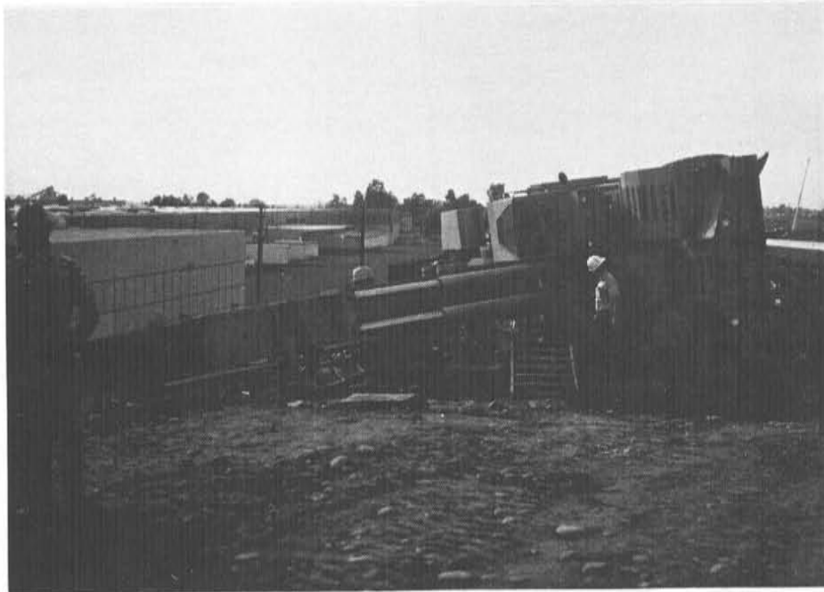
Figure No. 24 The Crane After Turning Over
