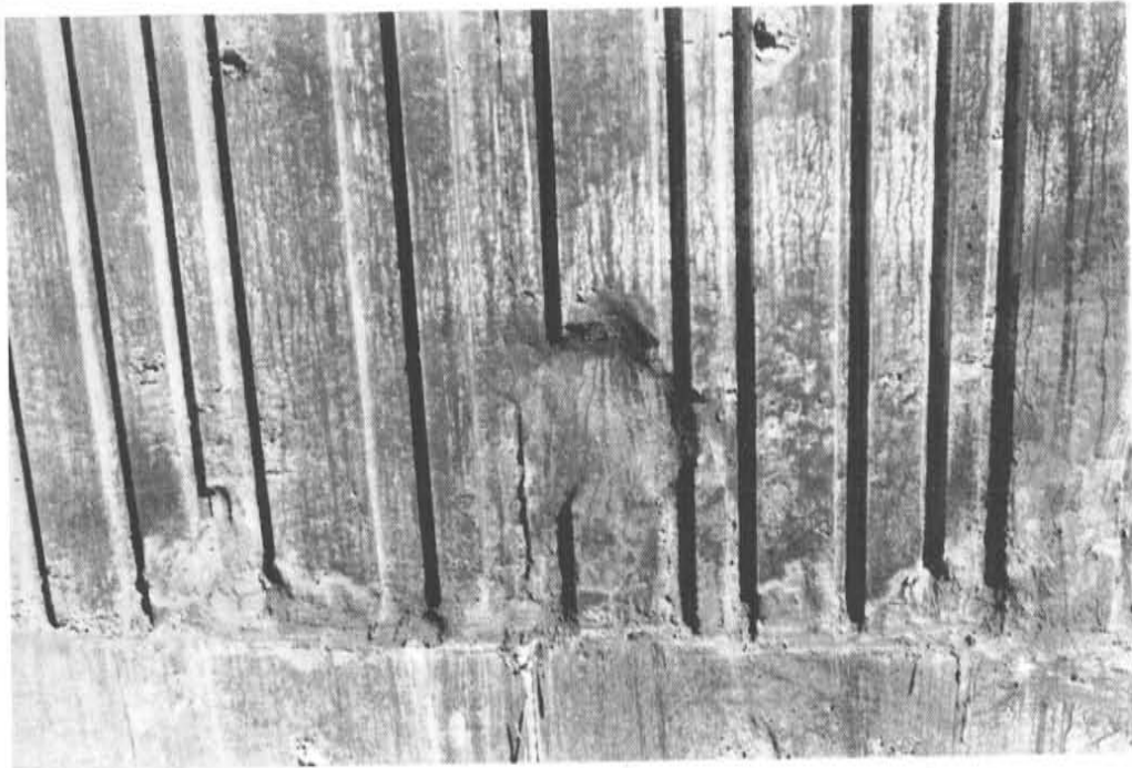
Figure No.29 Patching Attempts To Remedy The Severe Honeycombing
