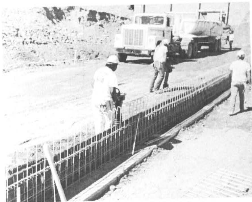
Figure No. 6 Trucks Dumping the Backfill Material and Workers are Compacting the 2 Foot Zone Area
