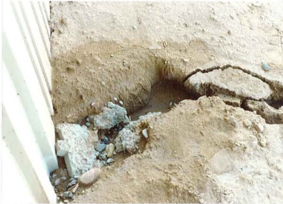
Figure 47 Erosion Channel Immediately Below Vertical Crack of the SE Wall.
