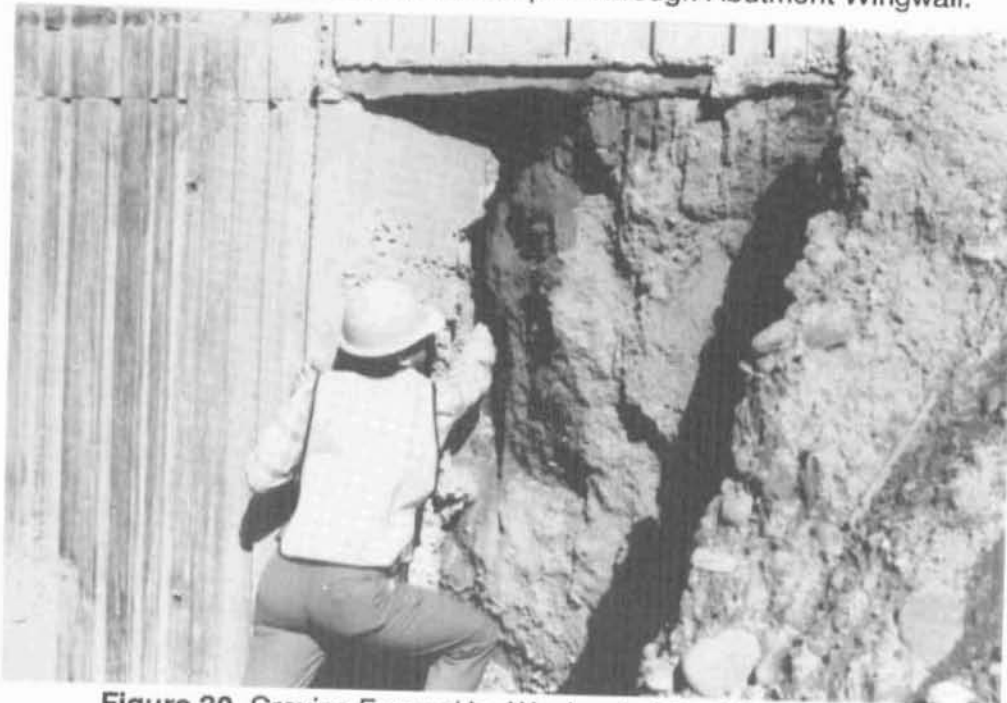
Figure 30 Crevice Formed by Washout of Backfill Material.
