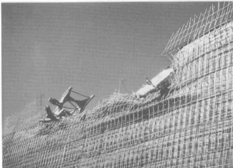
Figure 34 Damage Caused By Overturned Crane.
