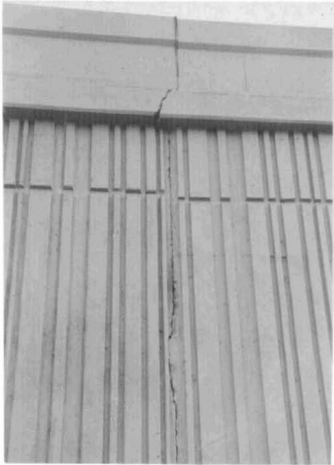
Figure 45 Vertical Crack at the Interface of the SE Wall and the Bridge Abutment.
