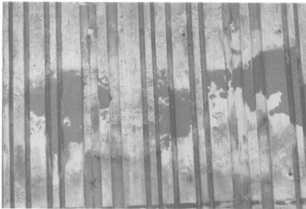
Figure 19 Honeycombing Was Still Visible After Patching Attempts.
