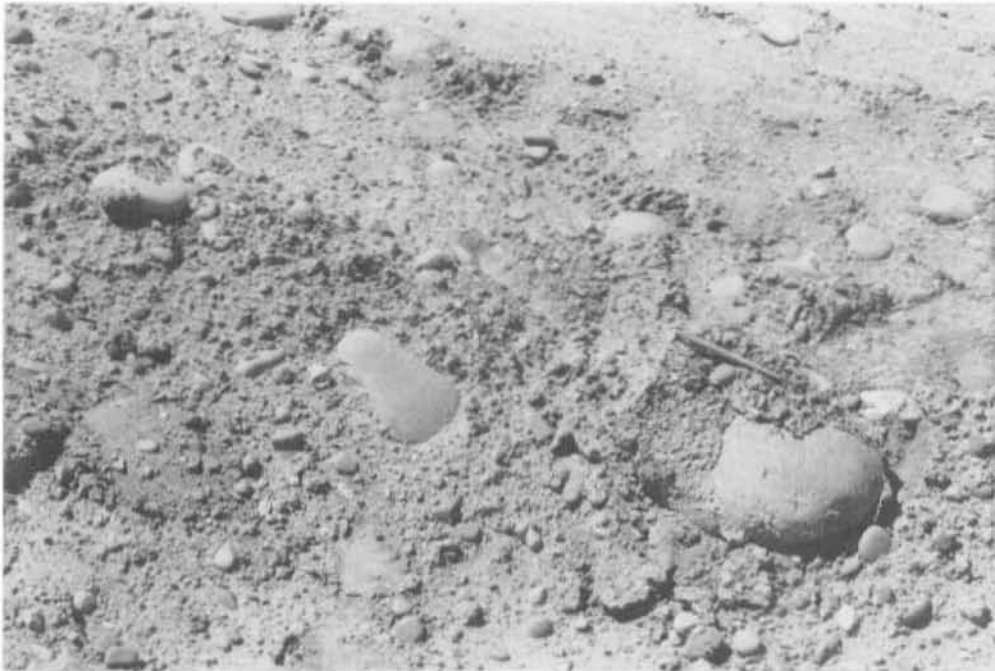
Figure 23 Backfill Material With Rocks Larger Than the 6" Sieve.
