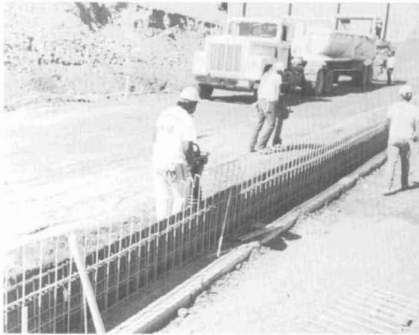
Figure 10 Dump Truck Used to Deliver Backfill Material and Hand Tampers Used for Compaction Near the Backing Mats.
