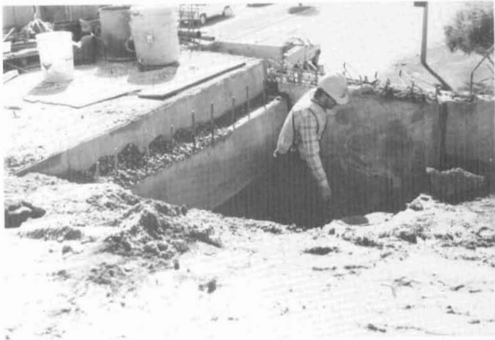
Figure 31 Void at the Top of the Embankment Due to Loss of Backfill Material.
