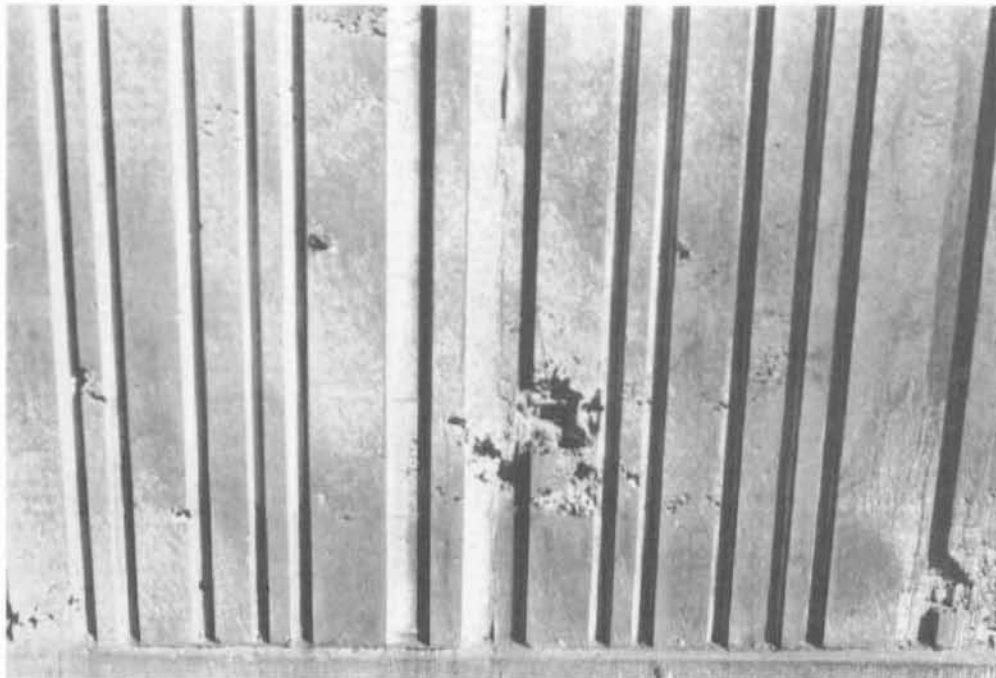
Figure 26 Exposed Reinforcing Steel Due to Severe Honeycombing.
