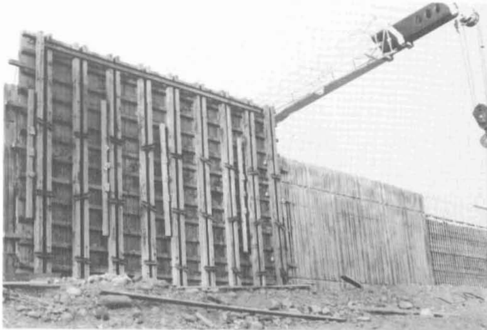
Figure 39 Forms of the SE Wall Were Placed Similarly to the Other Walls.
