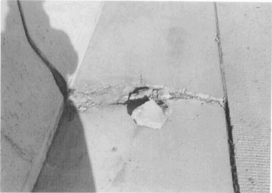
Figure 46 Damage to the Concrete at the Top of the Cracked Interface.
