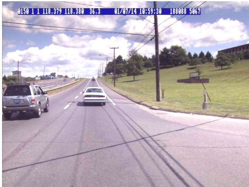
Location 118.37 km Mean IRI -11.05 m/km Transverse Reflection Cracking
