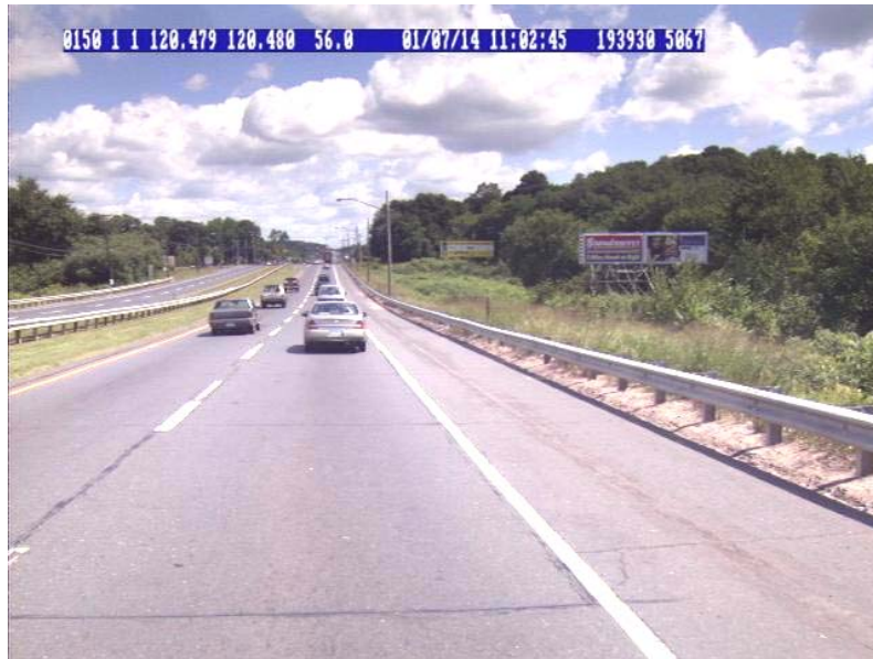
Location 120.48 km Mean IRI – 1.96 m/km Transverse and Longitudinal Reflection Cracking
