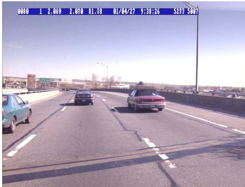
Location 2.08 km Mean IRI -7.27 m/km Rough Bridge Deck and Joints
