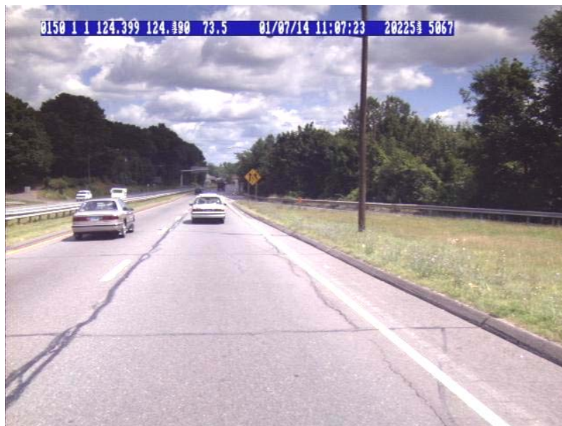
Location 124.40 km Mean IRI – 1.63 m/km Sealed Transverse and Longitudinal Reflection Cracks
