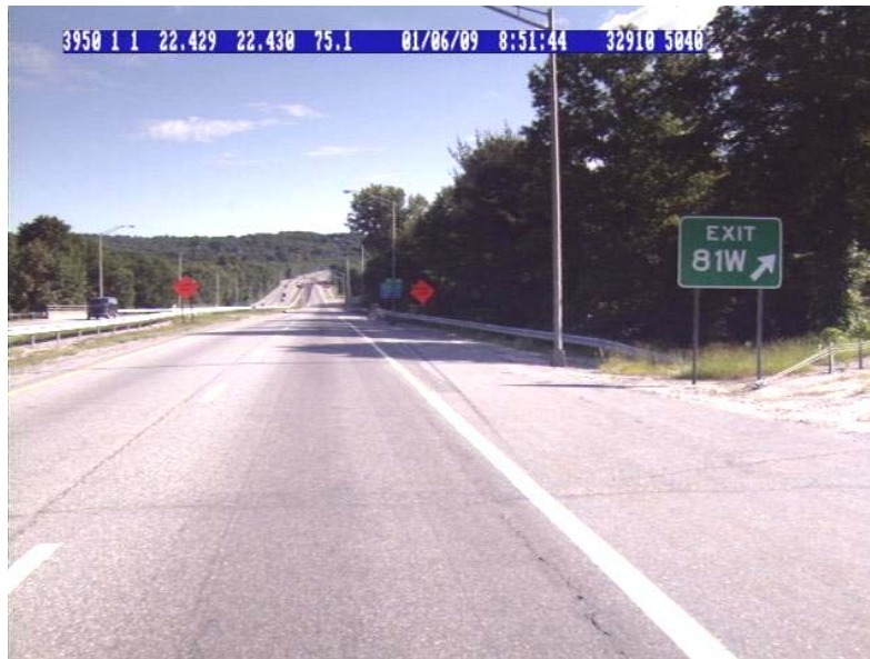
Location 22.43 km Mean IRI - 2.61 m/km Longitudinal Edge Cracking
