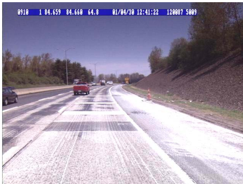
Location 84.66 km Mean IRI - 12.76 m/km Construction Project –Milling of Existing Bituminous Pavement
