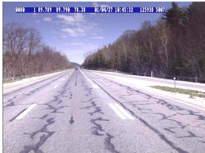
Location 89.79 km Mean IRI - 2.35 m/km Longitudinal Cracks in Wheelpaths
