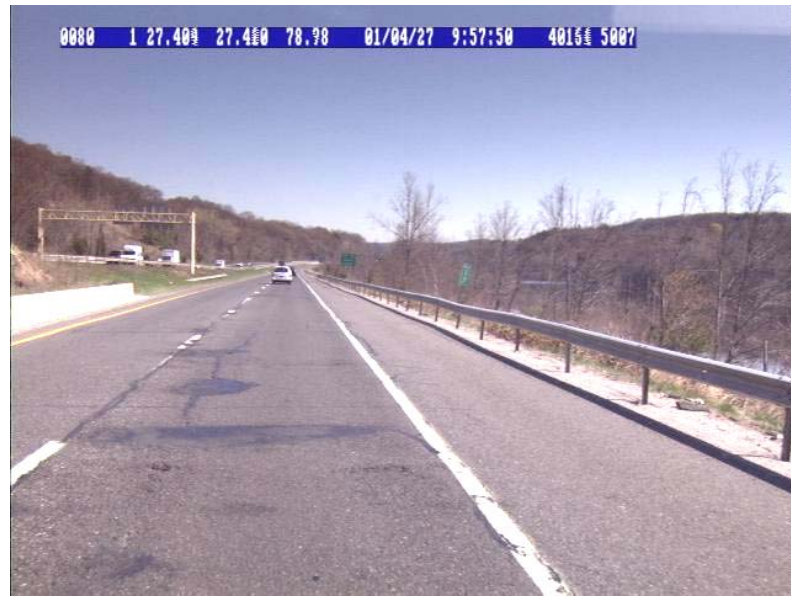
Location 27.41 km Mean IRI - 4.32 m/km Edge Cracking and Sealed Crack
