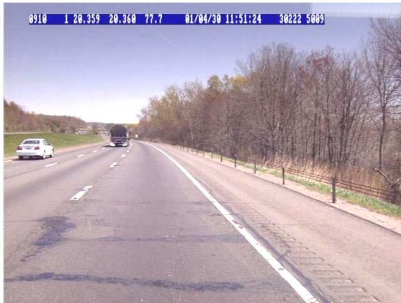
Location 20.36 km Mean IRI - 3.61 m/km Pavement Cracking
