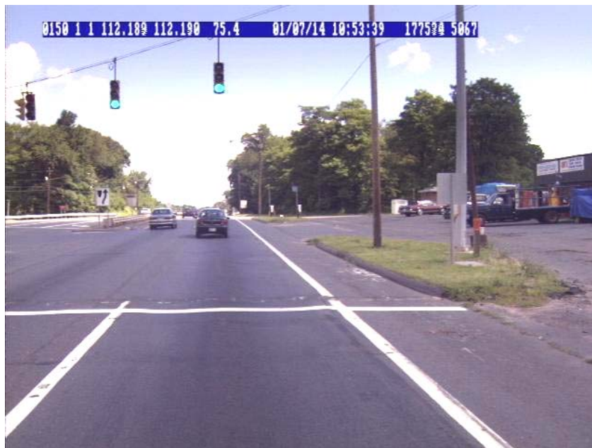
Location 112.19 km Mean IRI -8.28 m/km Rutted Pavement at Traffic Light
