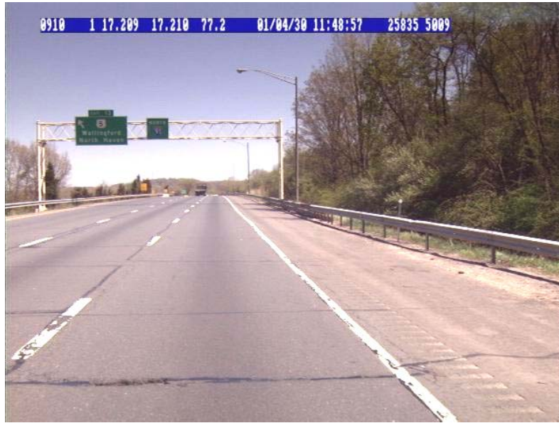
Location 17.21 km Mean IRI - 3.66 m/km Transverse Reflection Crack
