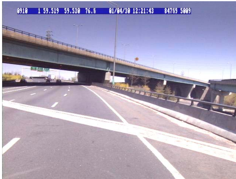
Location 59.53 km Mean IRI - 10.40 m/km Rough Skewed Bridge Joint
