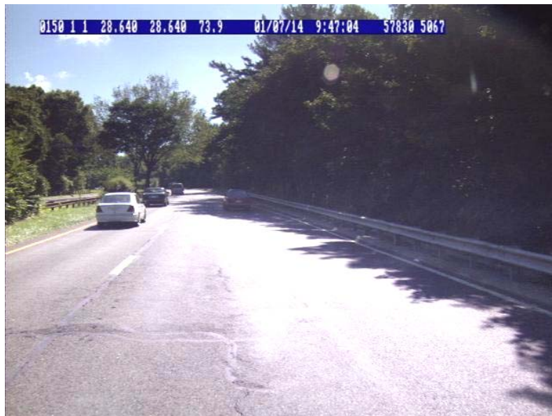
Location 28.64 km Mean IRI - 10.26 m/km Underlying Joint Distress
