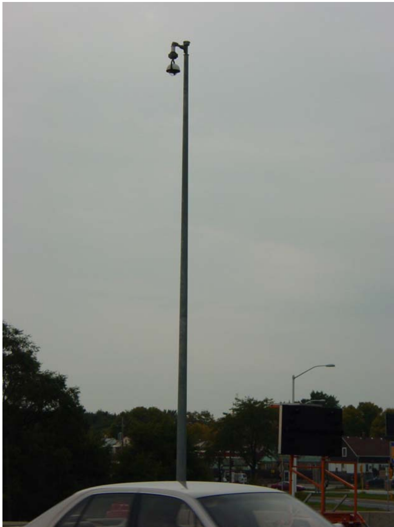
Figure 15-10: CCTV Camera Assembly
