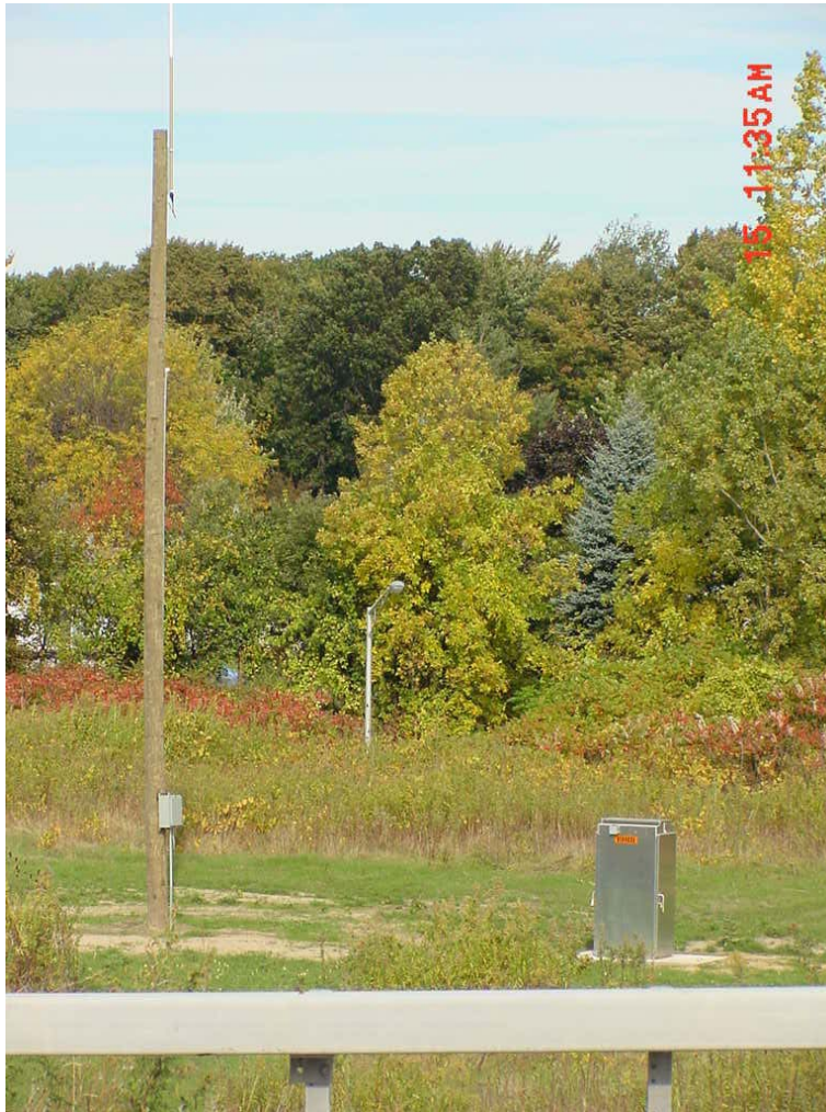
Figure 13-5: Highway Advisory Radio Station Along Freeway
