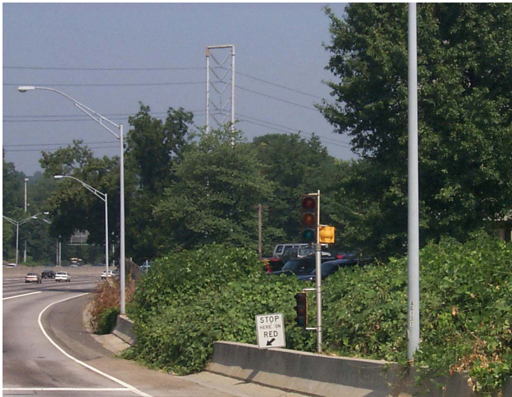
Figure 7-1: Ramp Metering Signals
