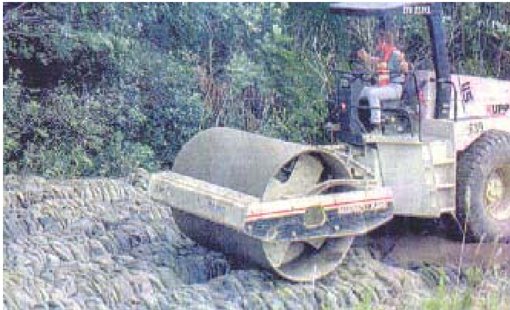
Figure B2. Construction of a Road Embankment Using Tire Bales as Subgrade
