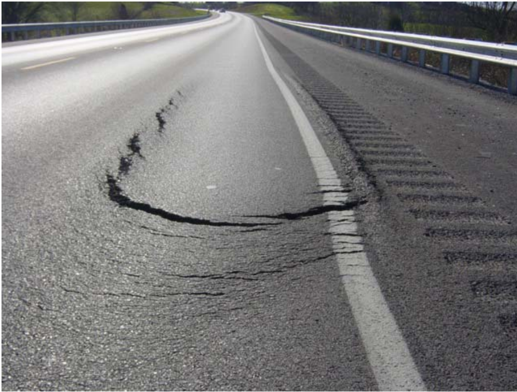
Figure 2.2 Slippage Cracking (View 2) [4]
