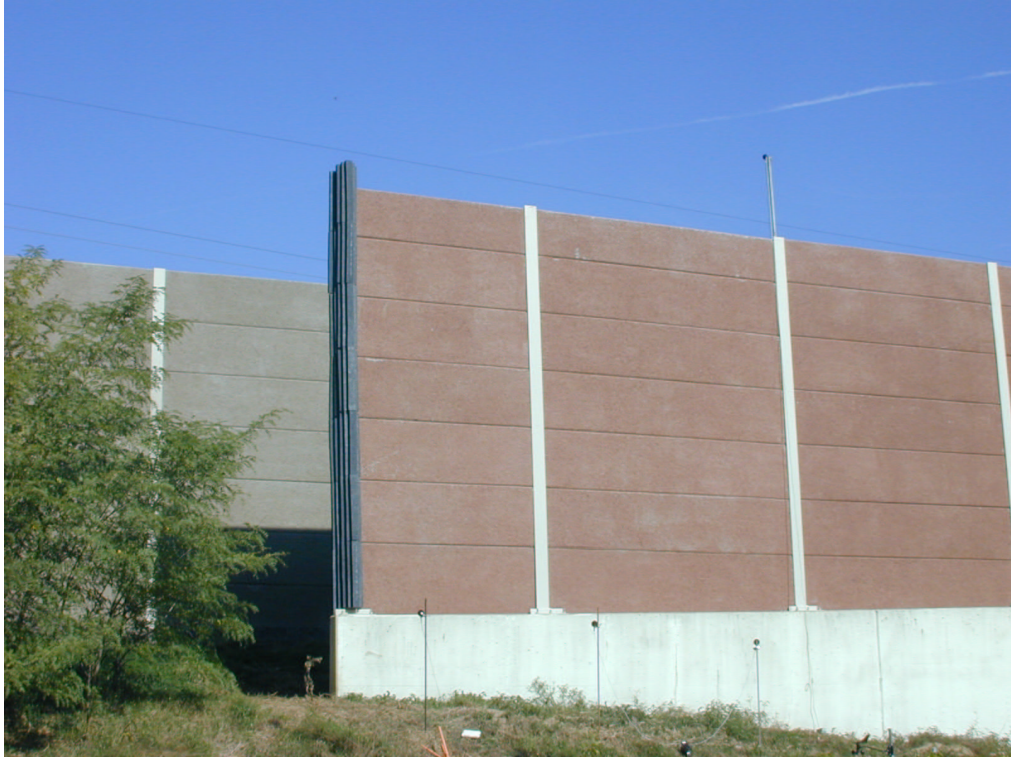
Figure 6.8. Installation of the absorptive QUASH treatment on the vertical edge of the barrier.
