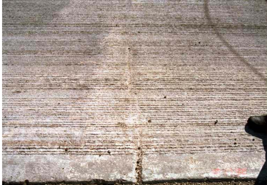
Figure 9. Surface Irregularity at the Shoulder Edge
