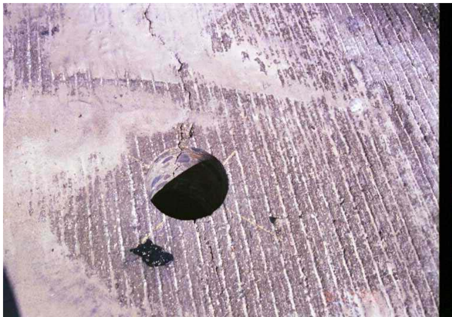
Figure 17. Core Hole - Longitudinal Crack
