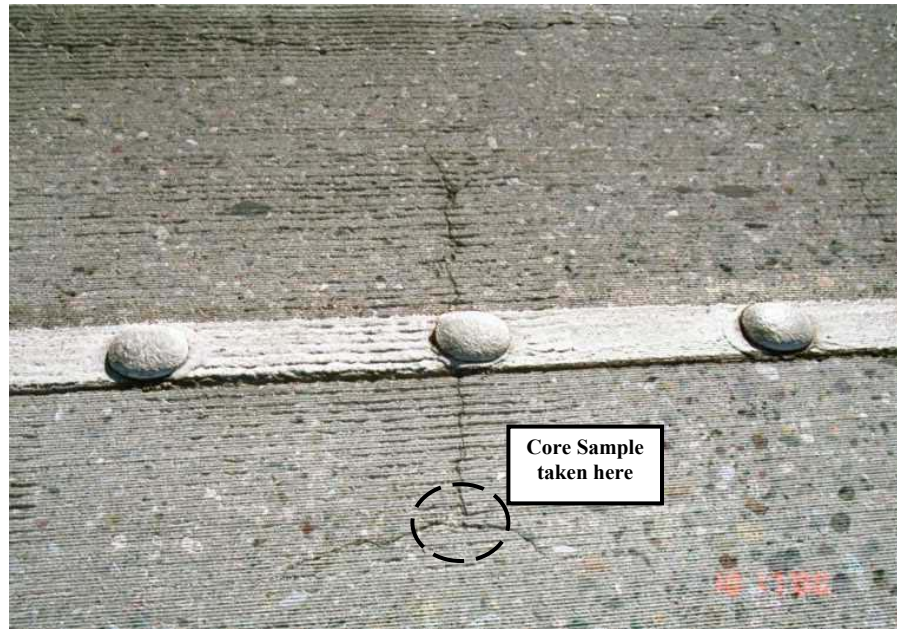
Figure 10. Crack across the Longitudinal Joint
