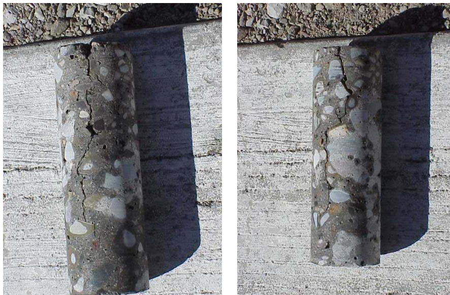
Figure 19. Core Sample - Longitudinal Crack
