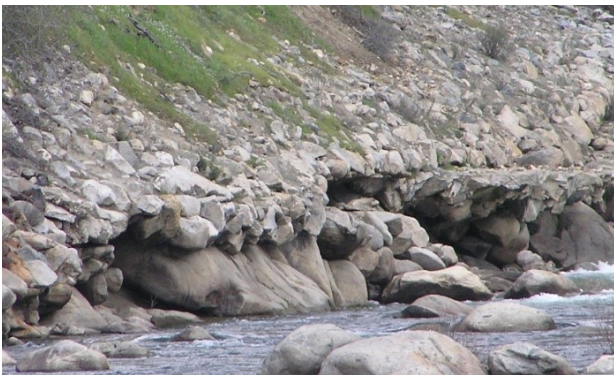
Toe of concreted RSP that has been undermined.
