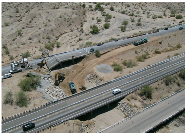
Bridge Abutment Failure at Tex Wash on I-10 after a Flood Larger Than the Design Flood
