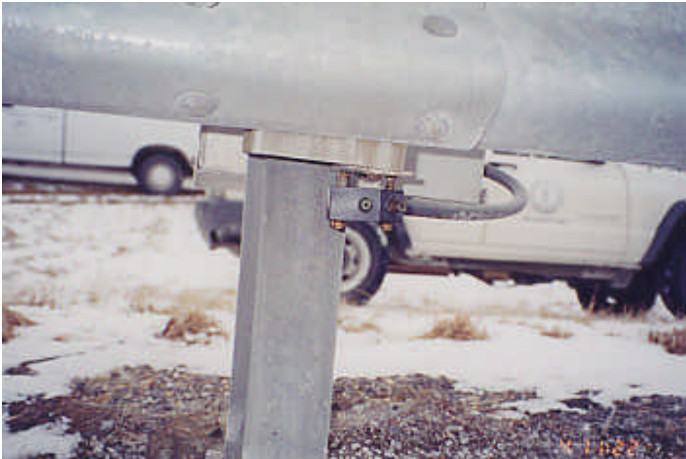
Figure 3. Spray Nozzle under Bridge Rail
