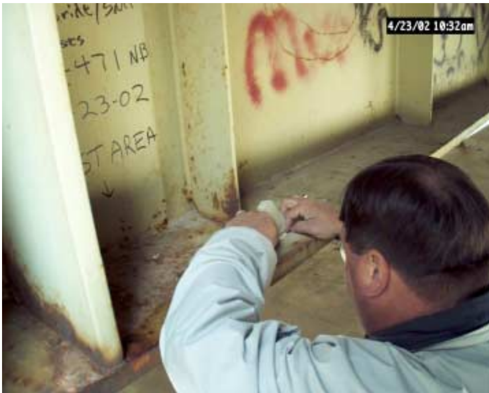
Figure 2 Technician installing sleeve on upper face of lower flange on floor beam (test area 1A).
