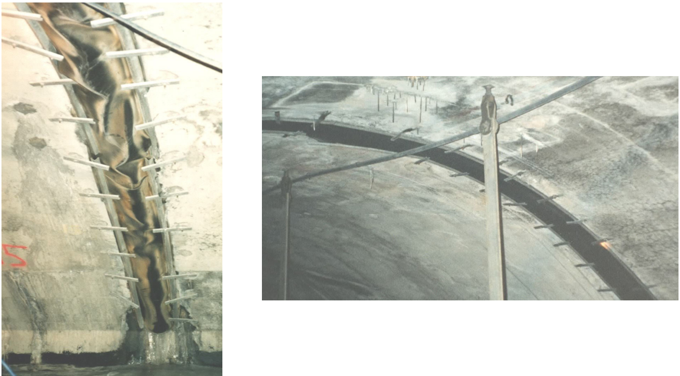
Figure 4.2 – Temporary drainage systems comprised of neoprene rubber troughs and 25 mm (1 in) aluminum channels.
