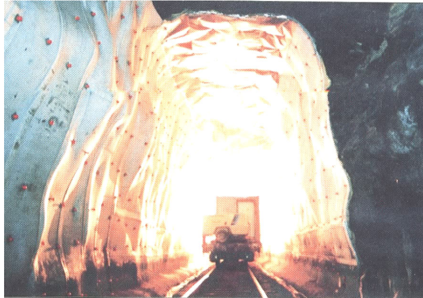
Figure 4.4 – Insulated panels used as a waterproofing lining to keep infiltrating water from freezing. (Photo courtesy of Tunnels & Tunnelling International)
