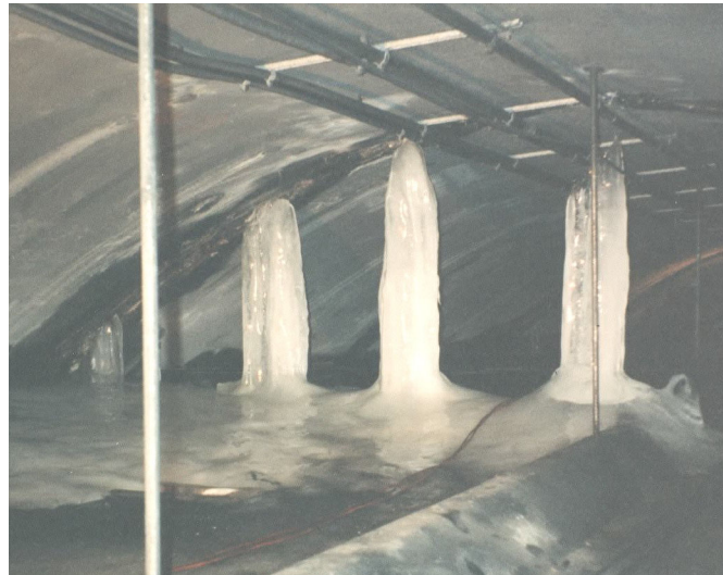
Figure 4.1 – Ice formation at location of water infiltration in plenum area above ceiling slab.
