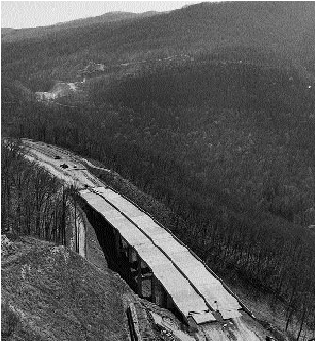
Earth slides halted construction in 1978 and in 1983, but the Commission on Transportation in the 21st Century funds helped complete this section of Route 23.
