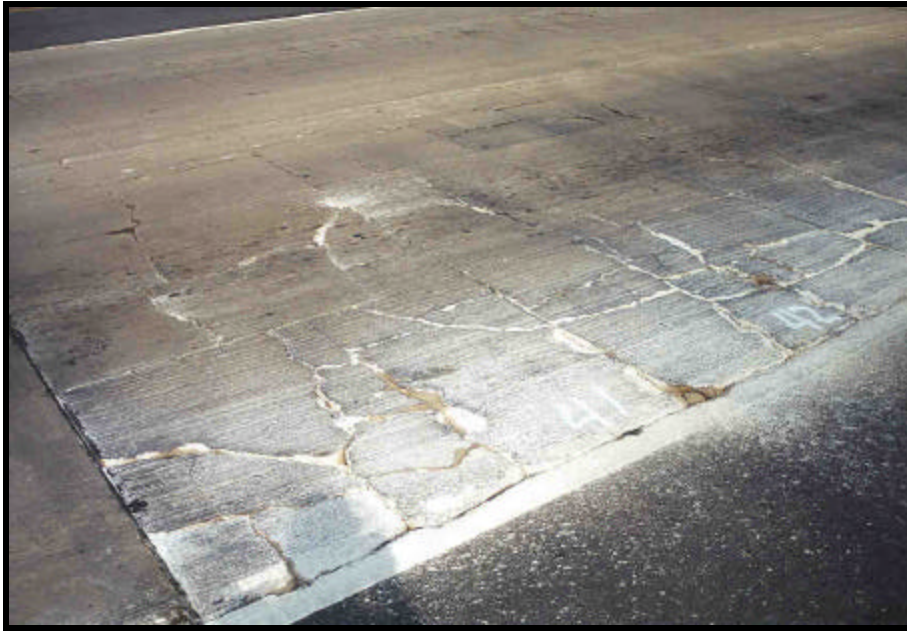
Figure 31. Area Of Significant Overlay Break-Up
