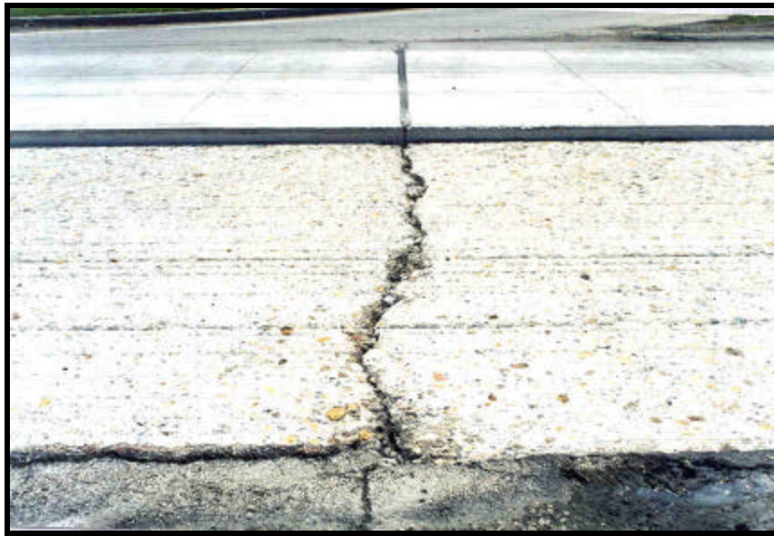
Figure 11. Severe Transverse Crack That Was Not Patched
