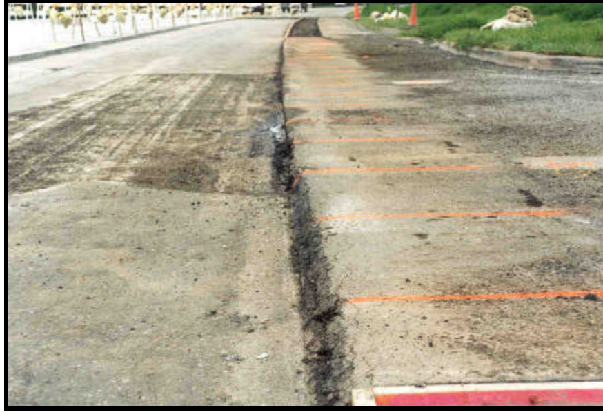
Figure 17. Worn-Down Pavement Edge
