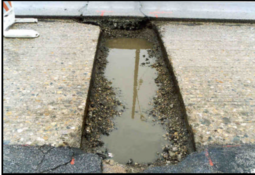
Figure 12. Rain Water Within A Patch Location
