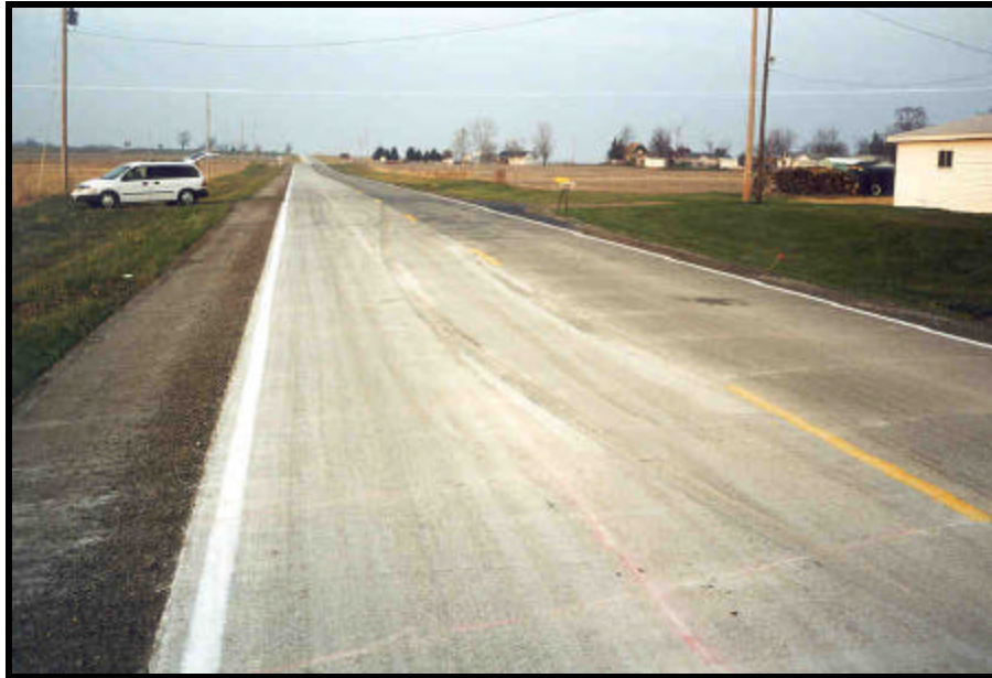
Figure 29. Tire Impression In Finished Concrete
