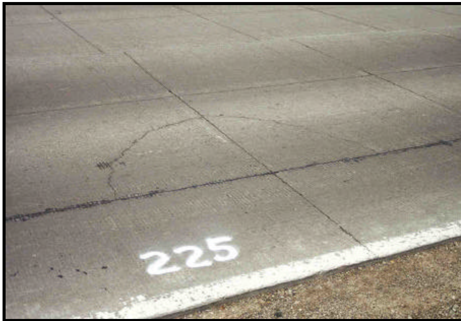
Figure 32. Panel Corner Break
