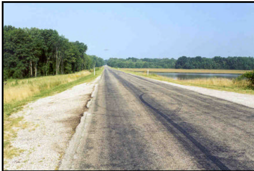
Figure 23. Original Pavement Edge Cracking
