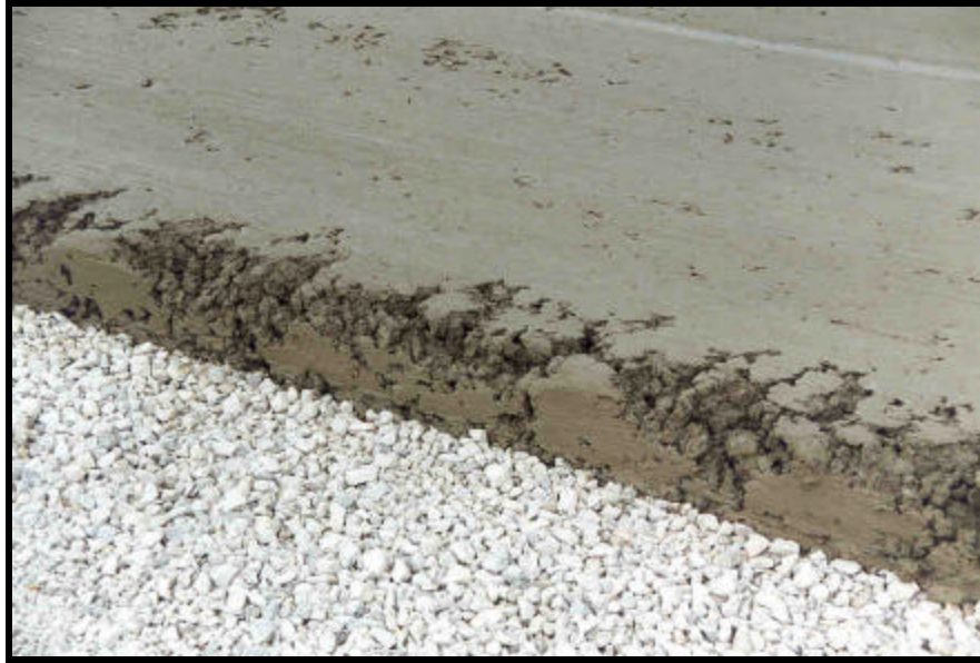
Figure 21. Honeycombed Appearance Of Concrete
