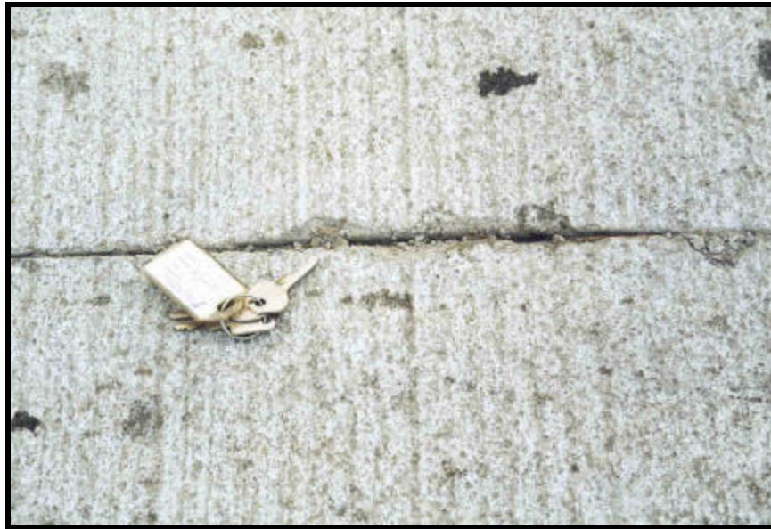
Figure 16. Tearing At A Partial-Depth Saw Cut
