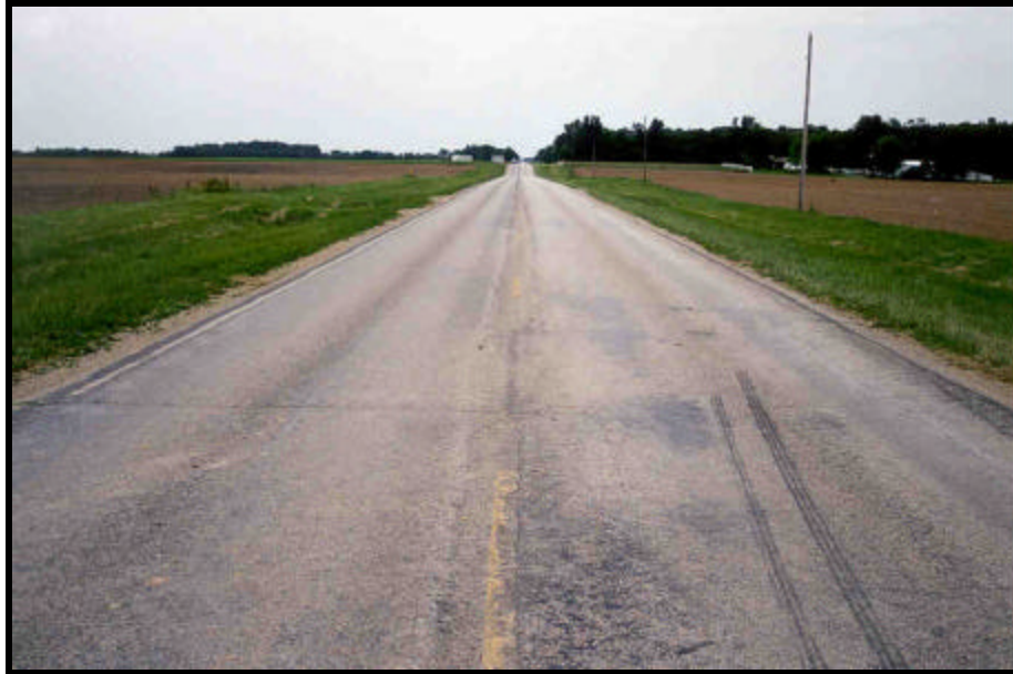
Figure 27. Existing Surface Distresses
