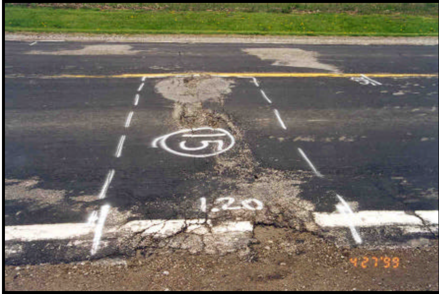
Figure 18. High Severity Transverse Crack
