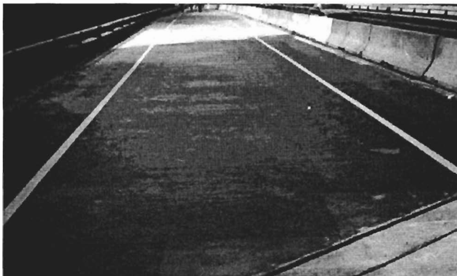
Figure 5.4. Outside lane and shoulder of Bridge 2 after MMLMC and ML overlay placement.
