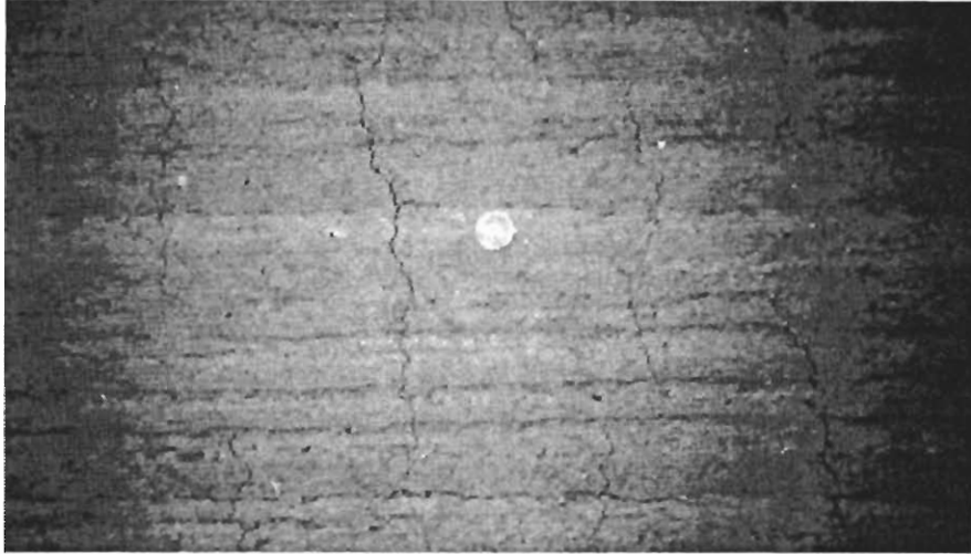
Figure 5.1. Plastic shrinkage cracking in Bridge 1R. The cracks are parallel with the axis of the rotating drums on the screed. The SF overlay was removed.
