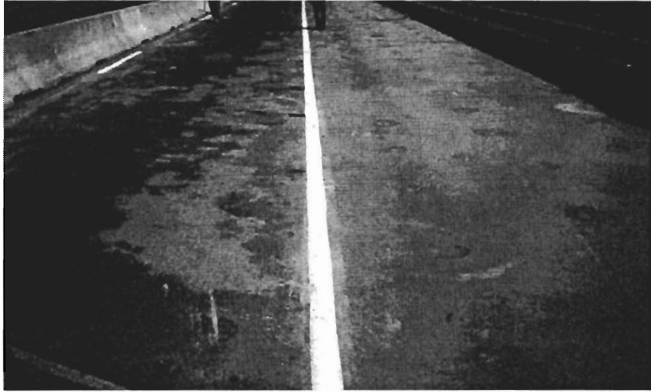
Figure 2.6. Bridge 6 prior to overlay placement. The Class I waterproofing was worn off much of the travel lane.
