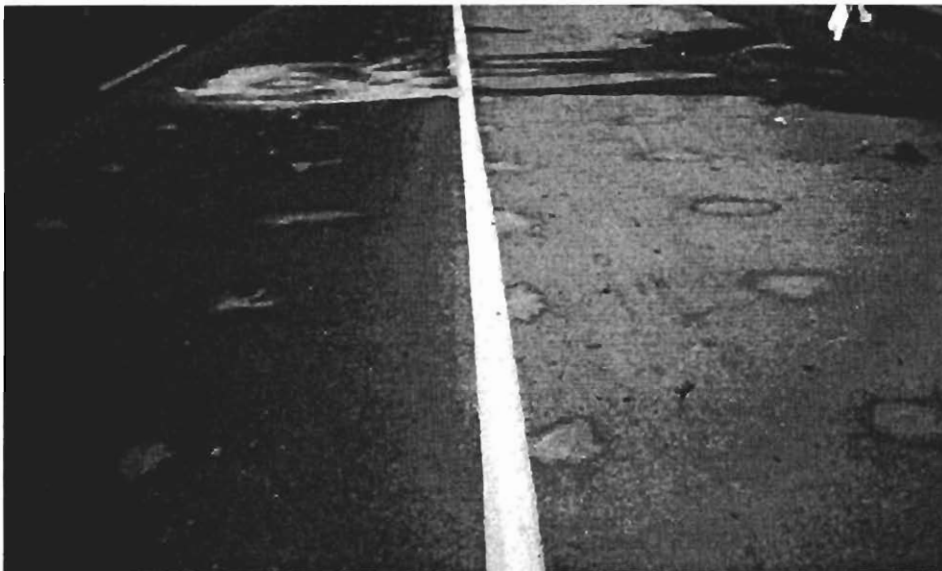
Figure 2.5. Bridge 4 prior to overlay placement. The wet spots are locations where half-cell potential measurements were taken.
