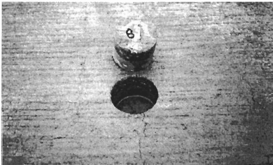
Figure 5.2. Bridge 1R after SF overlay placement. Core shows plastic shrinkage cracks are full depth.
