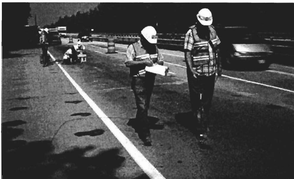
Figure 2.1. Measuring electrical half-cell potentials, foreground , and taking chloride ion content samples, background .
