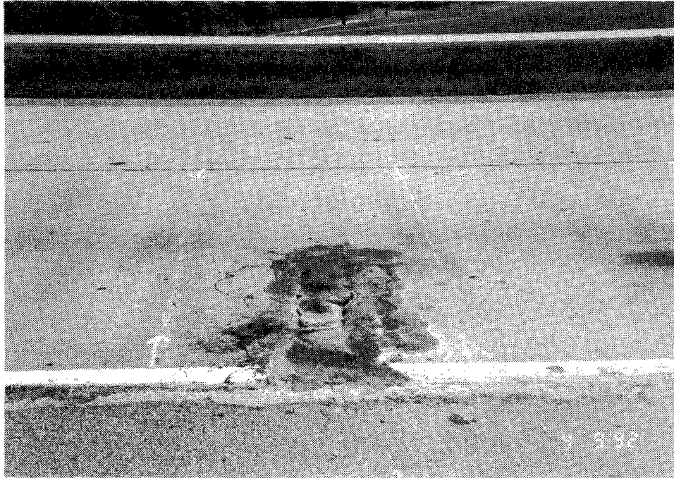
Figure 20. Marked out distress area.
