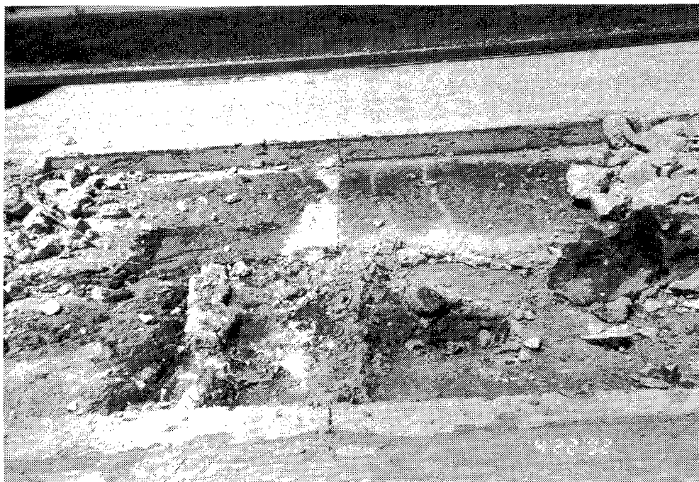
Figure 11. Movement of material caused by pumping.
