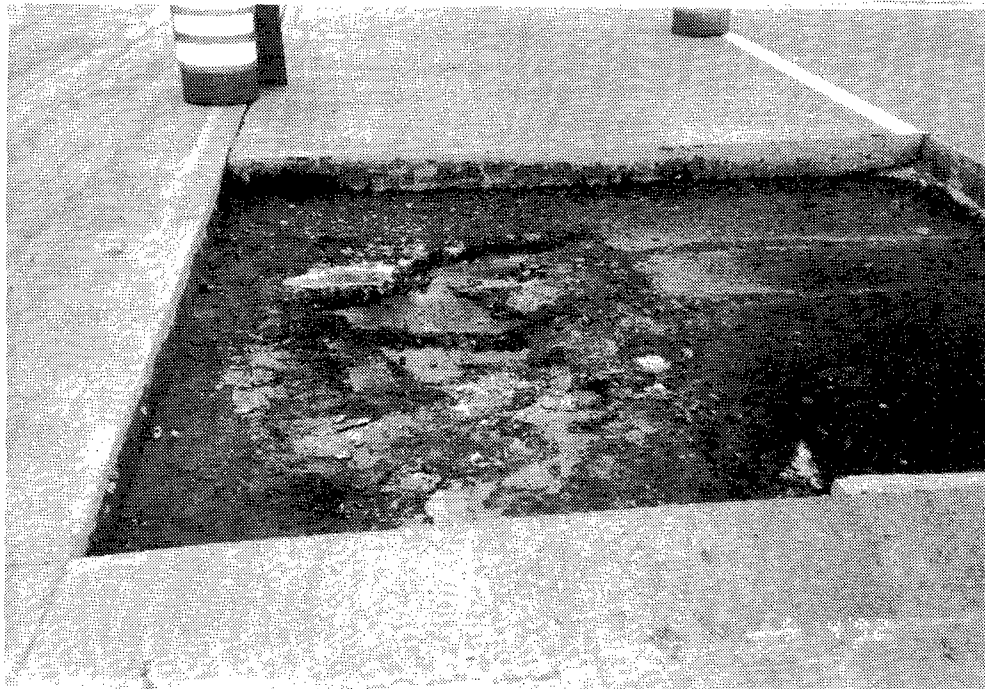
Figure 10. Erosion of subbase under punchout distress.
