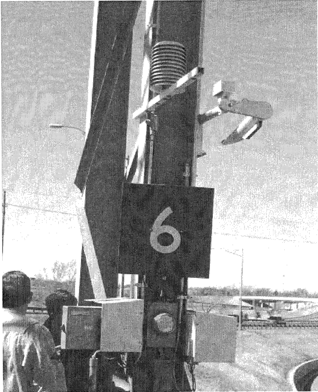
Figure D.4 Vaisala RPU in Amarillo
