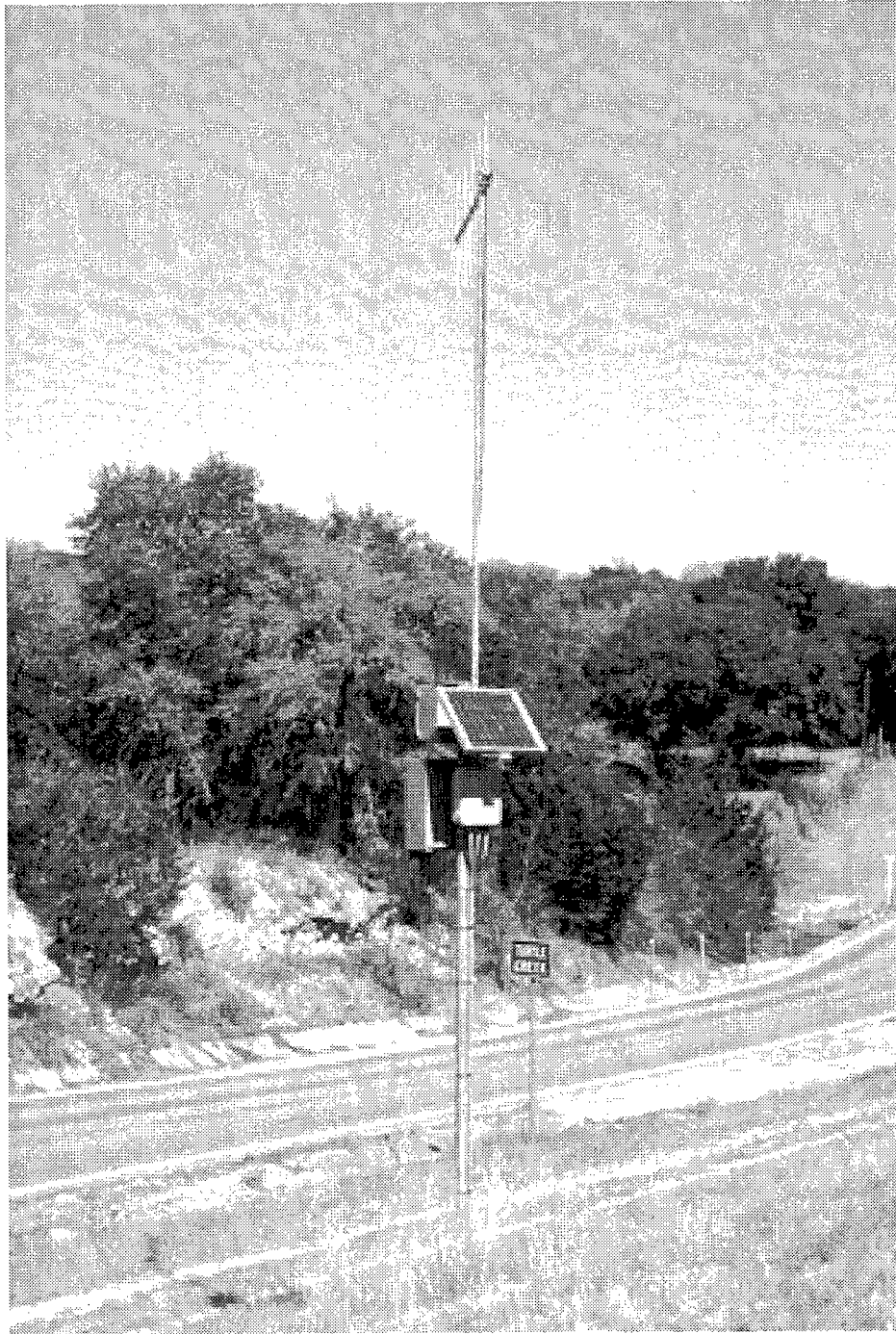
Figure D.1 ROS solar-powered RPU at Turtle Creek site in Kerr County
