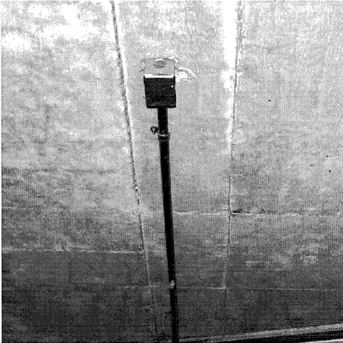
Figure D.2 Vaisala pavement sensor and conduit underneath bridge in Amarillo
