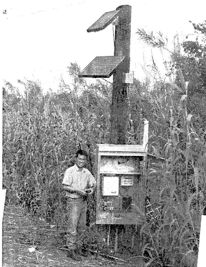
Figure 2.15 Aluminum cabinet and solar panel mounted on wooden pole
