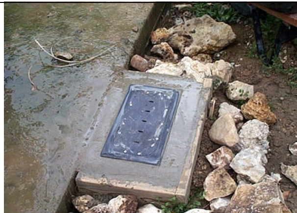
Non-boxed Effluent Sampler.
