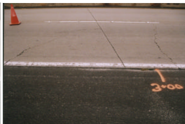
Figure 3.1.11 Corner break near approach joint at 06-CS1, Tracy Test Road (control section).
