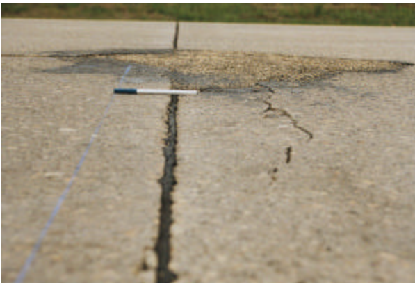
Figure 3.1.19 Close-up on transverse joint spalling at 19-3006.
