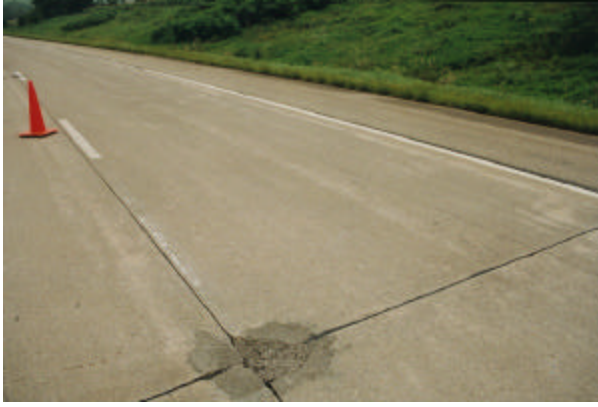
Figure 3.1.23 Corner break and repair at 27-4054.
