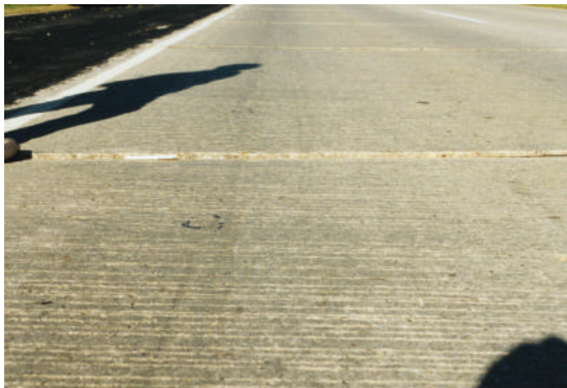
Figure 4.2.1 Faulted transverse joint in test section 55-3008.
