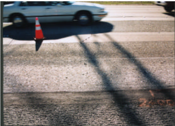
Figure 3.1.15 Transverse crack at test site 06-I-10 closer to leave joint.
