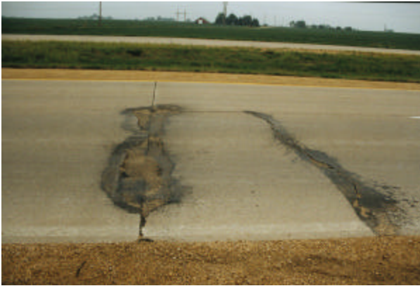
Figure 3.1.18 Typical transverse joint distress at 19-3006.
