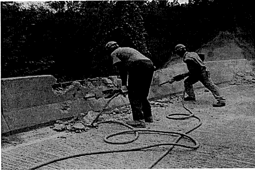
Figure 4. Concrete Removed From Parapet Using 90-lb Hammers
